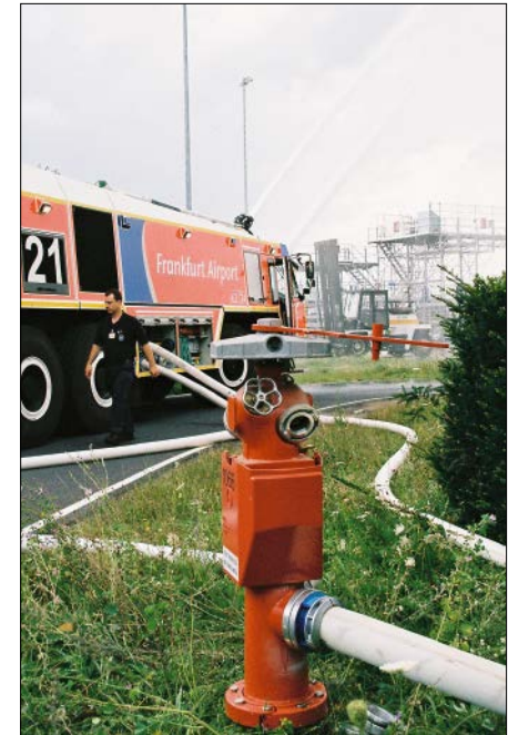
Fig. 7.8.5-02: Industrial hydrant for the supply of extinguishing water in industrial plants
