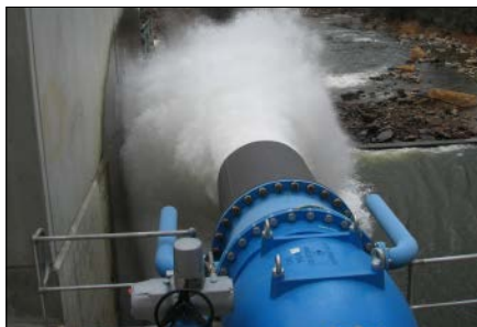
Fig. 7.6.3: Plunger valve DN 800, PN 10, with aeration as a bottom outlet valve in the wall of a dam
