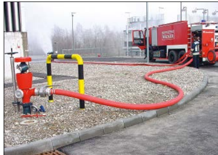
Fig. 7.8.5-01: Industrial hydrant for the supply of extinguishing water in industrial plants
