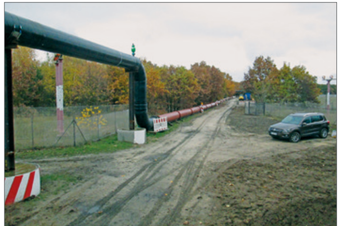
Pipe bridges in steel pipes maintain accessibility.
