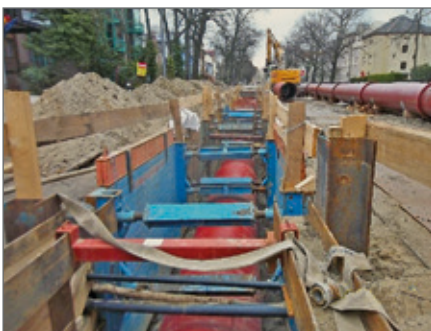
New DN 1200 GGG sewage pressure pipeline and DN 1000 GGG interim pipeline on the right.
