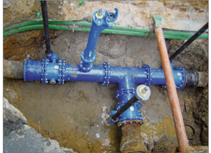
Safe and secure: installation of fittings and valves in buried pipeline construction.
