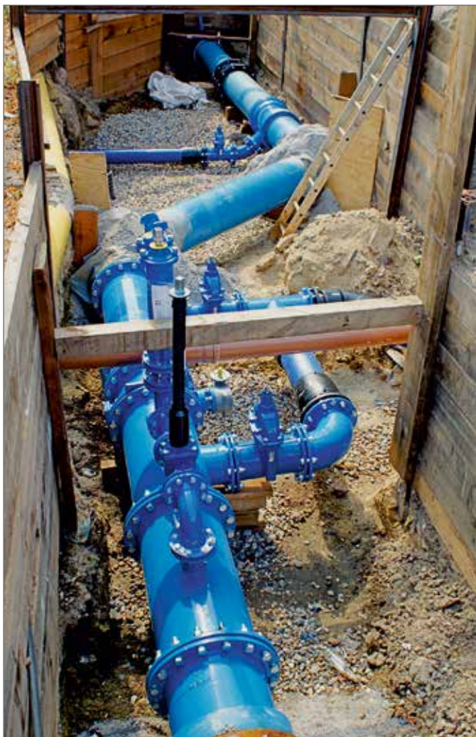
From time to time it was necessary to integrate valves and hydrants ...
