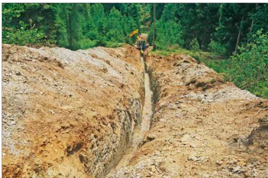
Carving the way downwards: the construction of the new wastewater pipe from the scattered settlements on the Guggenberg to the existing wastewater network was only possible with a hydraulic excavator with walking legs and a winch securing device.
