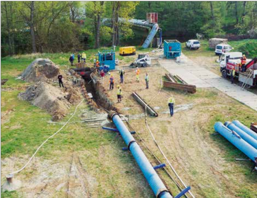
In the background: the ageing drinking water pipeline routed across the Nežárka bridge; in the centre: starting pit and the pipe string ready and waiting to be pulled in.
