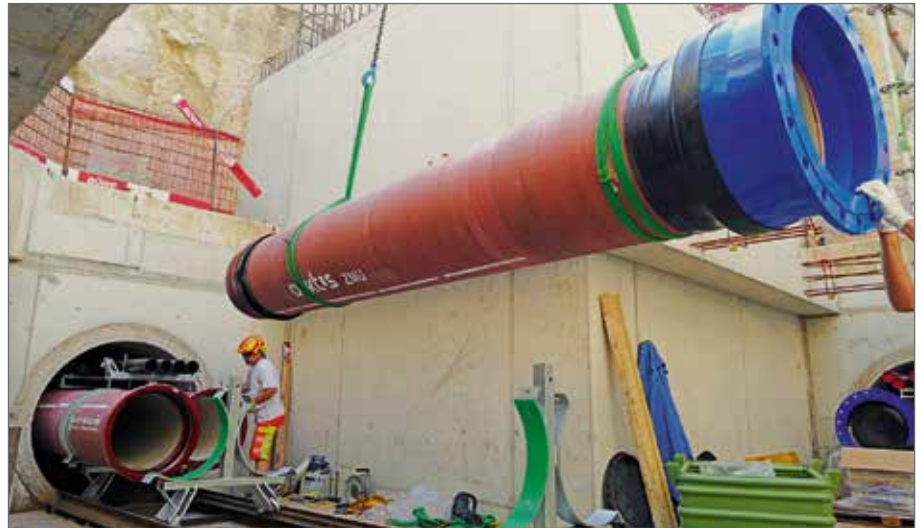
The very narrow space conditions on the installation side of the tunnel. Pictured here: the placing of a pipe on the transport clamp.
