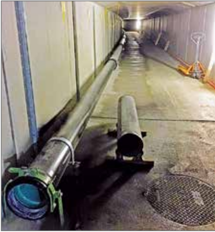
Extinguishing water pipeline along the service duct.
