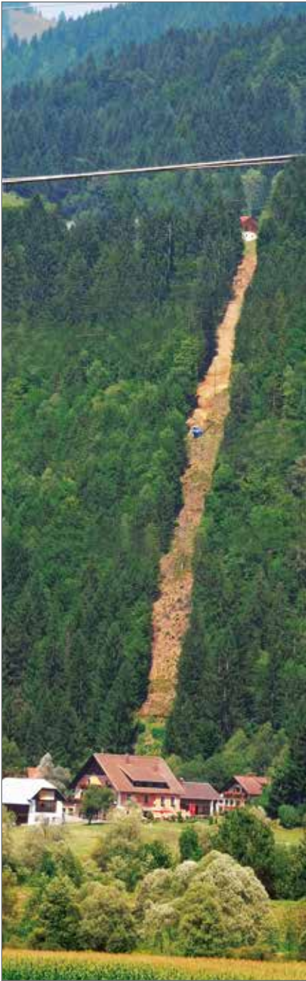
The 1.5 km long section of the wastewater pipeline climbing up the steep gradient. Because of its striking blue colour, the excavator can be spotted on the aisle through the forest.
