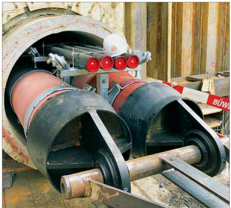
Arrival at the target shaft. The extremely tight space conditions in the microtunnel are clear to see.
