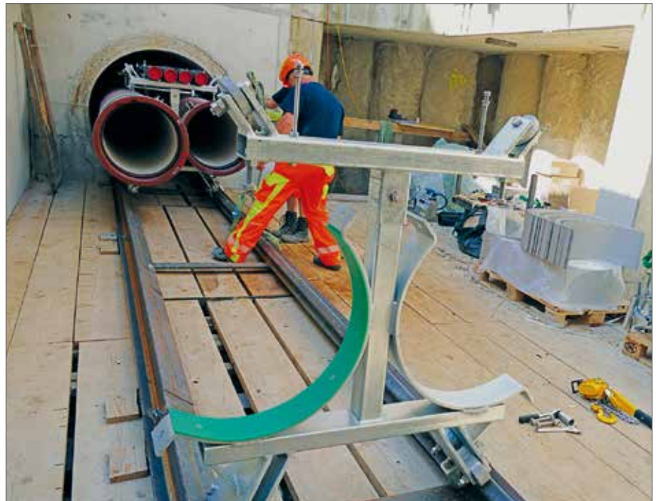
Pulling-in of two cast iron pipes simultaneously using specially developed mobile double pipe clamps.
