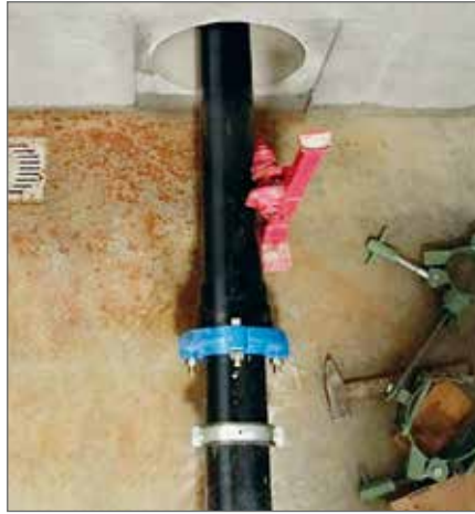
Branch pipeline from the service duct into the hydrant chamber.
