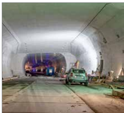
Completed service bay in the middle of the tunnel. Source: Bundesamt für Straßen (ASTRA), Switzerland
