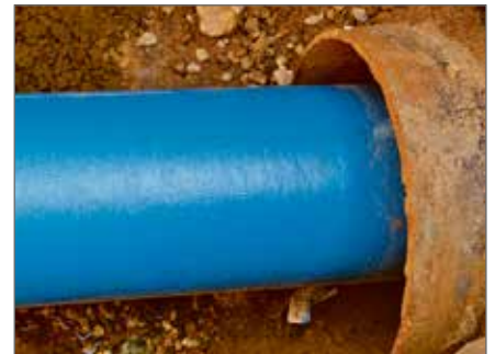
The pipe-string was pulled 6 m into the old pipeline in each case, dragging on the sheet steel cone.
