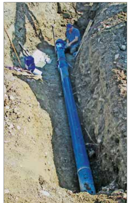
On grounds of the long working life and the quality of the material, Feldkirchen decided in favour of ductile iron pipes from Tiroler Rohre GmbH in nominal sizes DN 100, DN 125, DN 150 and DN 200.
