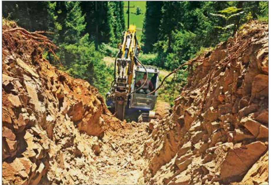
The „spider“ not only dealt with the earth-moving work but it also transported the pipes.
