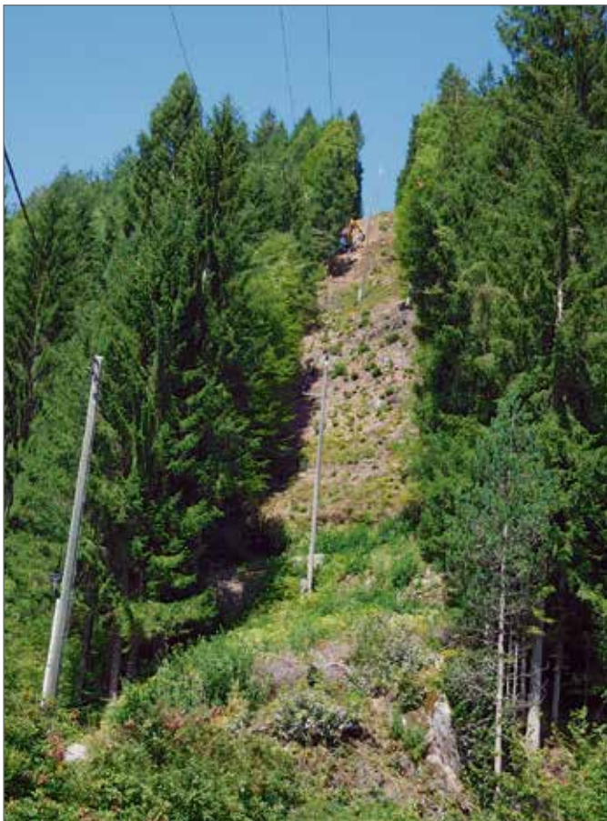
In order to protect ductile iron pipes against external factors, pipes with cement mortar coating were used. Delivering the usual pipe-bedding material on the steep slope was not possible.
