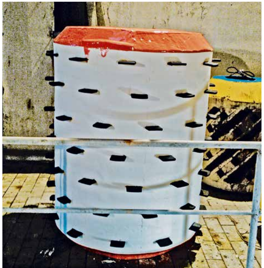
Very time-consuming: intensive pipe cleaning by pig (for each pipe the team worked 24-hours-a-day for four days).
