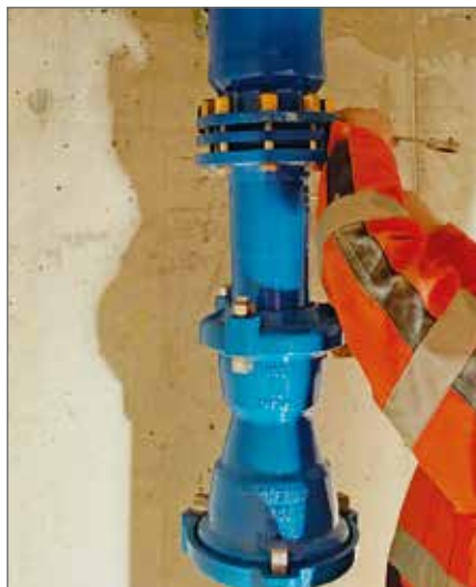
Assembly of a hydrant base VARIO 2.0 on the riser in the hydrant chamber.
