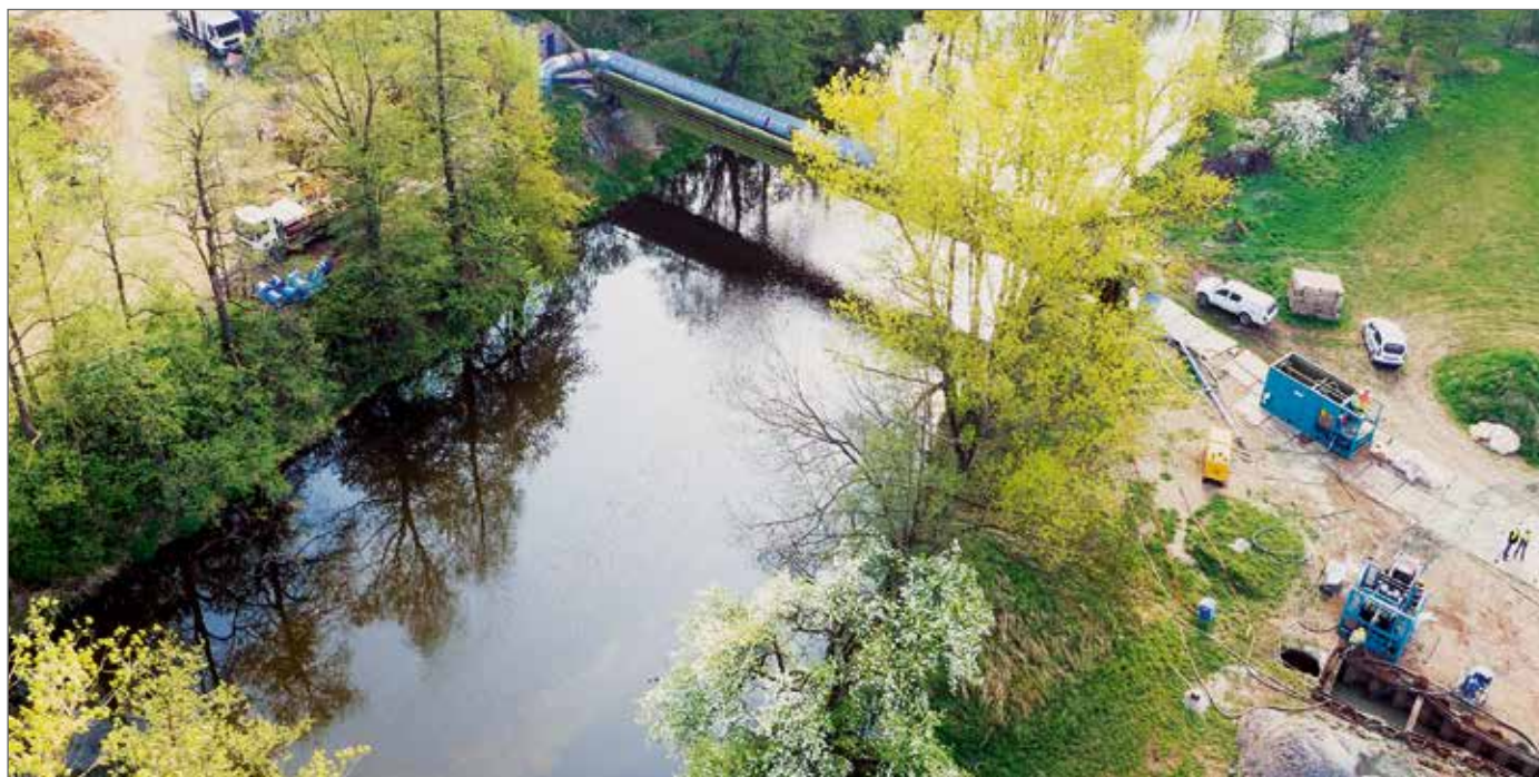
A view over the construction site to the right and left of the Nežárka.
