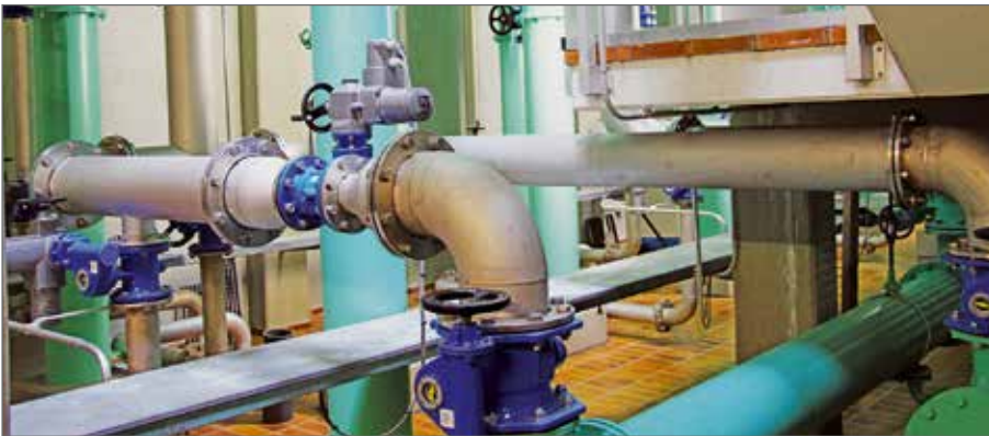
PAS10 adaptor and spacer, ERHARD ROCO wave butterfly valves with integral electric drive.
