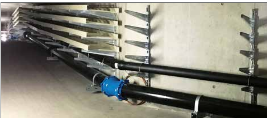
A bend in the pipeline route secured with a restrained joint Fig. 2806.
