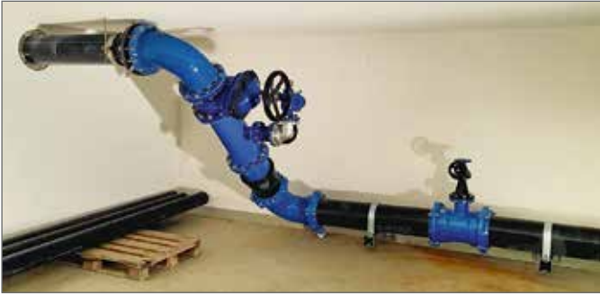
Connection of the extinguishing water pipeline in the "Engi" portal with pipeline valve, cleaning facility and vent valve.
