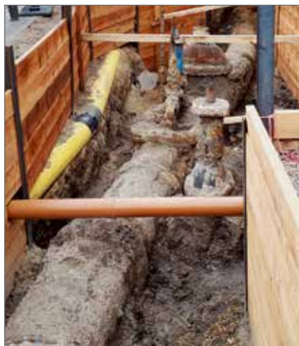
After 120 years of operation, the DN 700 grey cast iron pipeline is in a very passable state of maintenance.
