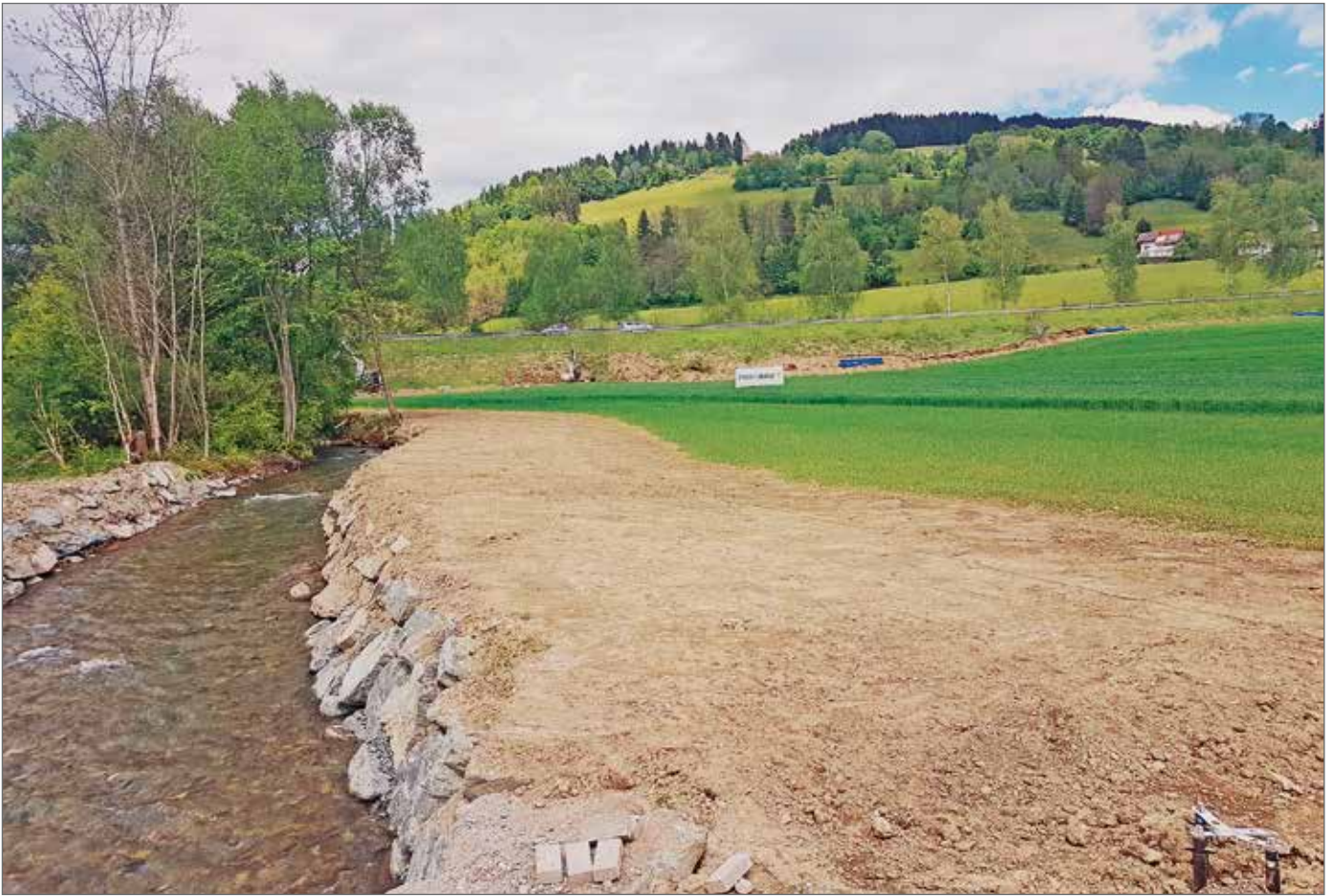
A few stream crossings had to be made in the course of the construction work. A problem here was the fast rise in water levels on site shortly after a period of bad weather with heavy rainfall.
