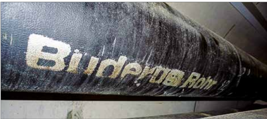
Ductile iron pipes inside the Rhine culvert.
