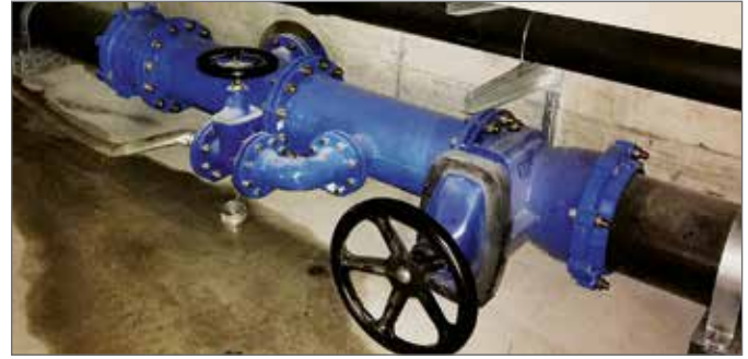
Pipeline shut-off valve, drainage and cleaning connections and lateral outlet to branch pipelines for hydrants.
