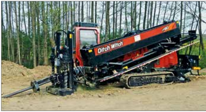
With a "Ditch Witch JT60", between the bore was widened in stages to 400 mm, 500 mm, 700 mm and finally to 950 mm.
