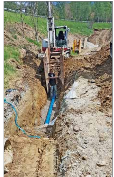
5,750 m cast iron pipes from Tiroler Rohre GmbH have been installed in the last three years. They replace the ageing PVC pipes.
