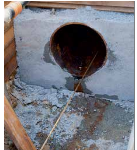
Pulling the new pipe into the existing old pipeline using the pull-in technique.
