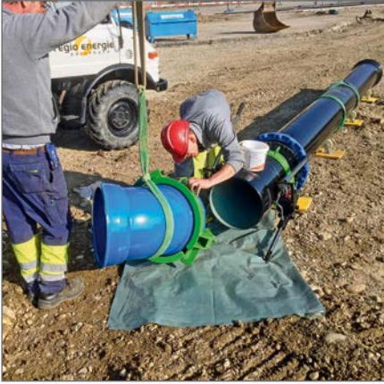
Preassembly of an ECOFIT DN 400 double-socket bend outside the trench profile with hydraulic pipe-laying equipment
