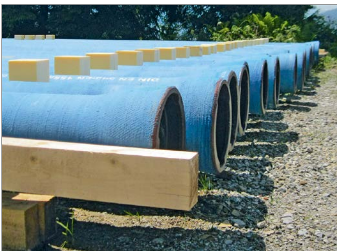
The store of ductile iron pipes ready for transport and installation by helicopter
