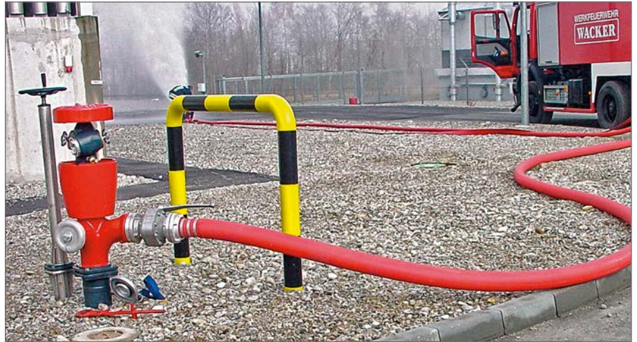
Industrial hydrant for extinguishing water supply on industrial premises
