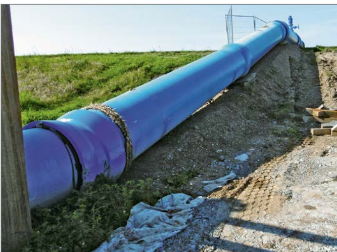
The route of the DN 800 interim pipeline over the dike between the pipe bridge over the River Mulde and the Canitz waterworks
