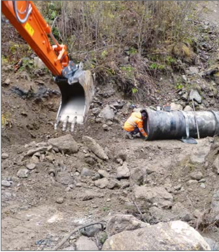
After the storm: expensive repairs for restoring the pressure pipelines
