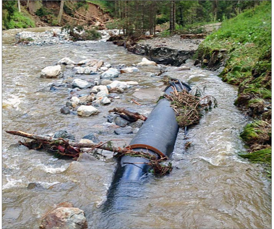
The storm caused the destruction of numerous pressure pipelines in the Sölk valley in Austria. Conventional, non-restrained push-in joints did not withstand the extreme loads.
