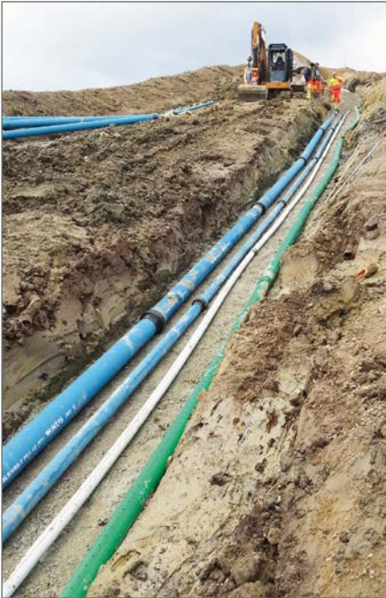
Installation of the ductile turbine and supply pipelines in the same trench
