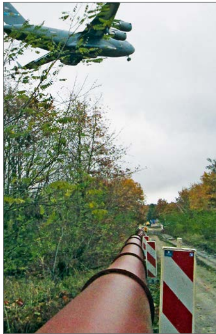
Interim pipeline along the route of the sewage pressure pipeline to be renovated in the approach path to Berlin Tegel Airport
