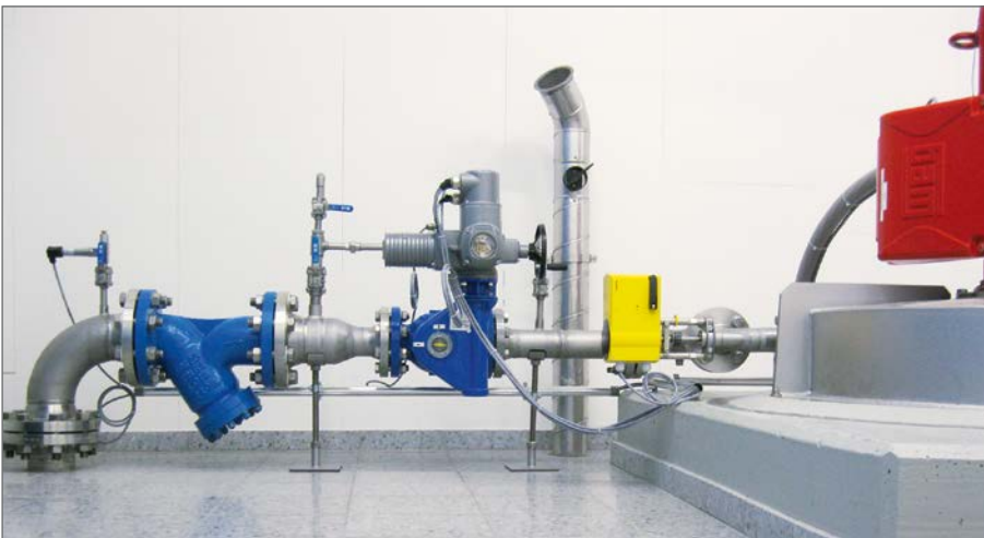
Connection of the turbine pipeline to the turbine with a dirt trap and a ball valve, each in PN 64
