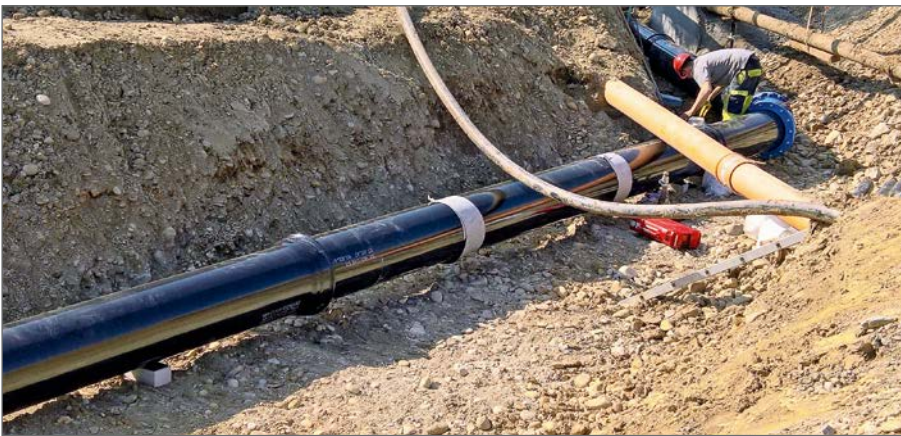
Assembly of the new DN 400 transport pipeline made more difficult because of the need for it to run beneath factory supply pipelines
