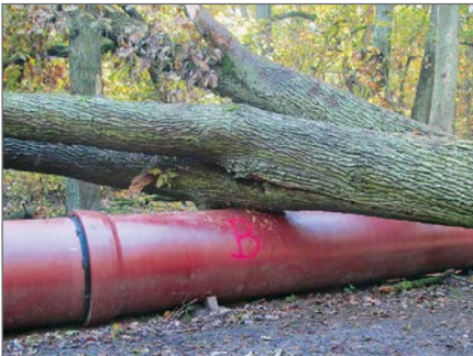
An uprooted oak tree which fell onto the interim pipeline did not result in any operational disruptions
