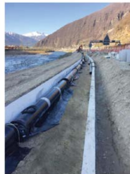
The route of the drinking water pipeline between the Ticino River in the Swiss Canton of the same name and the A2.
