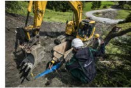
Assembling the pressure pipeline with VRS®-T restrained push-in joints in the pipe trench
