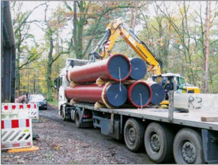
The 6 m long pipes are delivered direct to the construction site by truck
