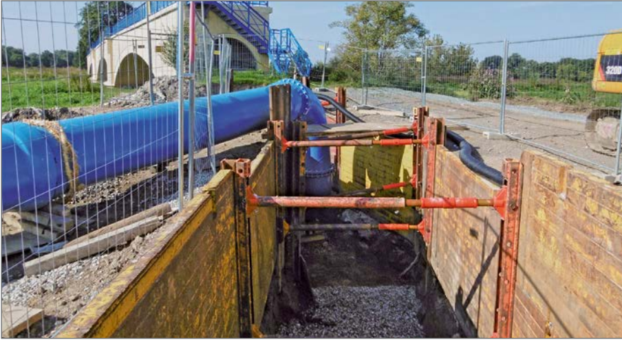
Excavation pit with a DN 800 interim pipeline coming out of it and onto a pipe bridge over the River Mulde
