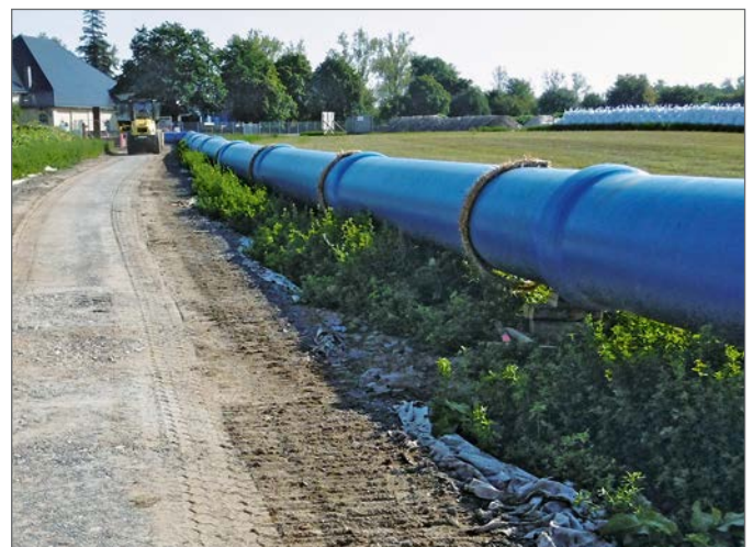
The straight section of the interim pipeline along the construction road to the Canitz waterworks
