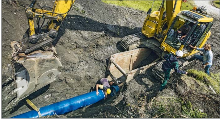
The progress is remarkable: The team from Rumpf Bau install and assemble 5 to 6 ductile iron pipes a day.
