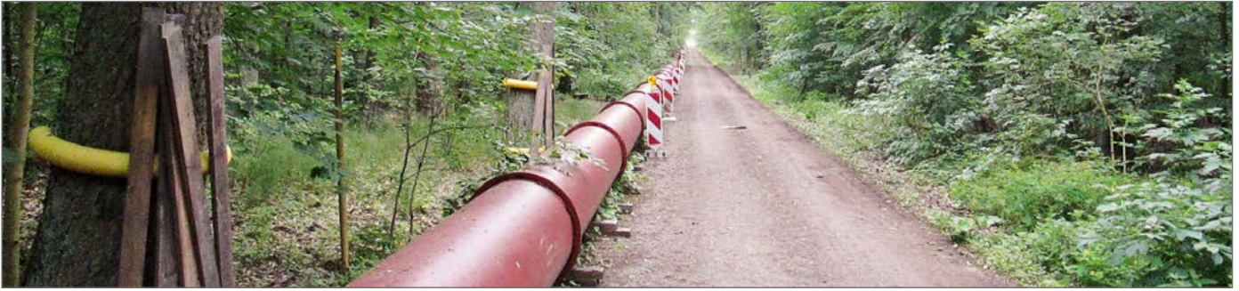
Environmentally friendly and space saving construction of the interim pipeline along a forest road
