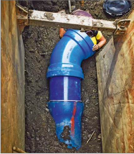
Fittings are also used in the construction of the power plant pipelines.
