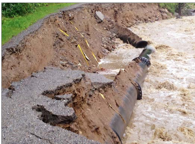
A power station pipeline installed next to a stream bed; once exposed by the scouring water, the non-restrained socket joints were pulled apart.
