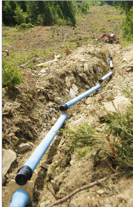
Ductile iron pipes flown in by helicopter, ready for assembly from bottom to top
