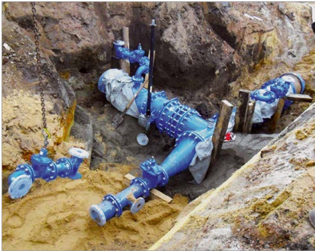
Figure 3: Valves and fittings in ductile cast iron in the DN 150 range – Wiener Straße
