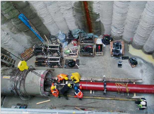
Figure 5: A view down into the launch pit during assembly of the traction head
