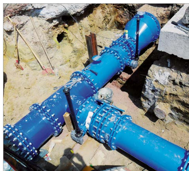
Figure 2: DN 500 valves and fittings in ductile cast iron – Wiener Straße
