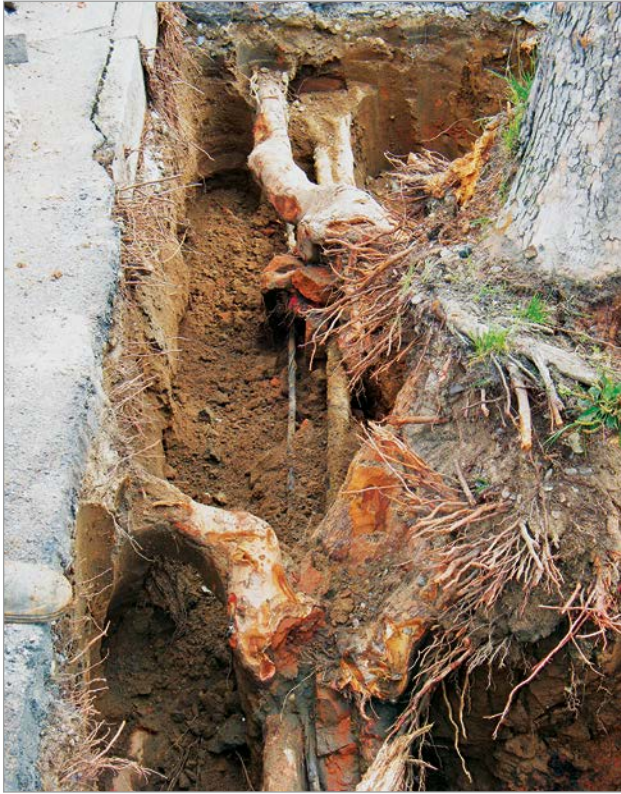
Figure 1: Tough roots in the utility trench of a telecommunications line
