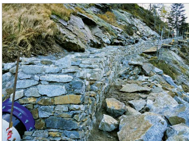
Figure 8: Almost natural reconstruction with a quarry stone wall around the pressure pipeline
