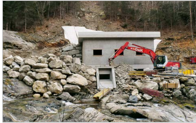
Figure 13: Power plant building with an underground channel to return the water to the Tomé mountain stream
