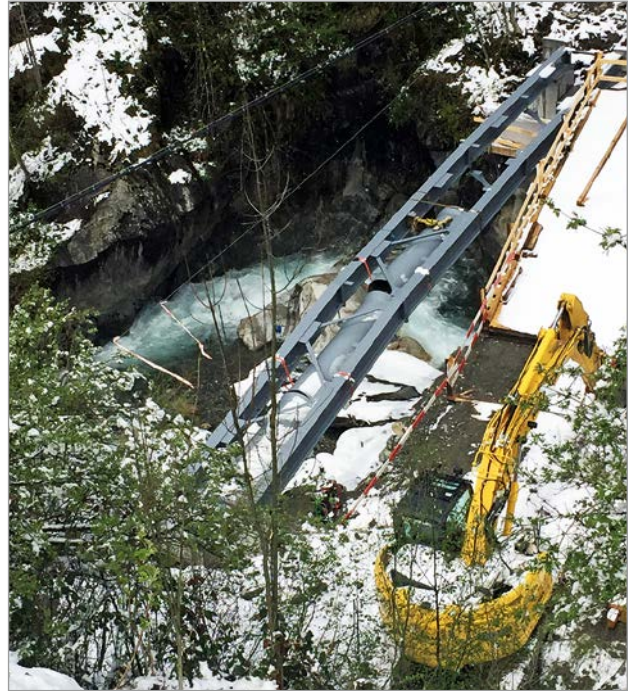
Figure 7: Steel construction of the footbridge with pre-assembled DN 1000 cast iron pipes underneath the bridge
