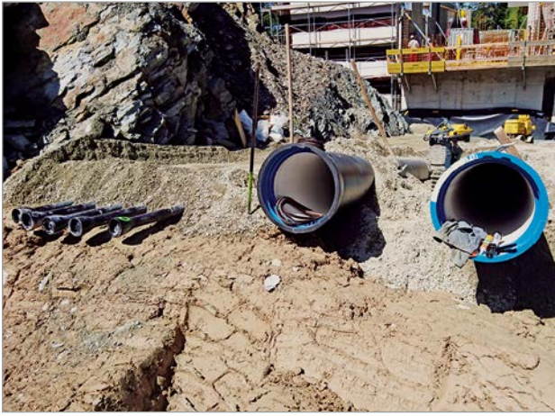
Figure 1: Ductile iron pipelines – five DN 80 reservoir pipelines and two DN 600 extraction pipelines
