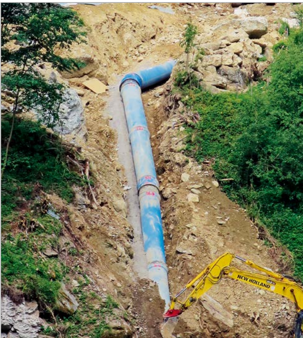
Figure 6: Backfilling the pipe trench and restoring the surface in difficult Alpine terrain
