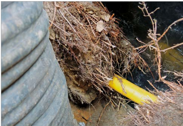
Figure 2: Fine roots in the utility trench of a gas pipeline Source: Heidger, C.
