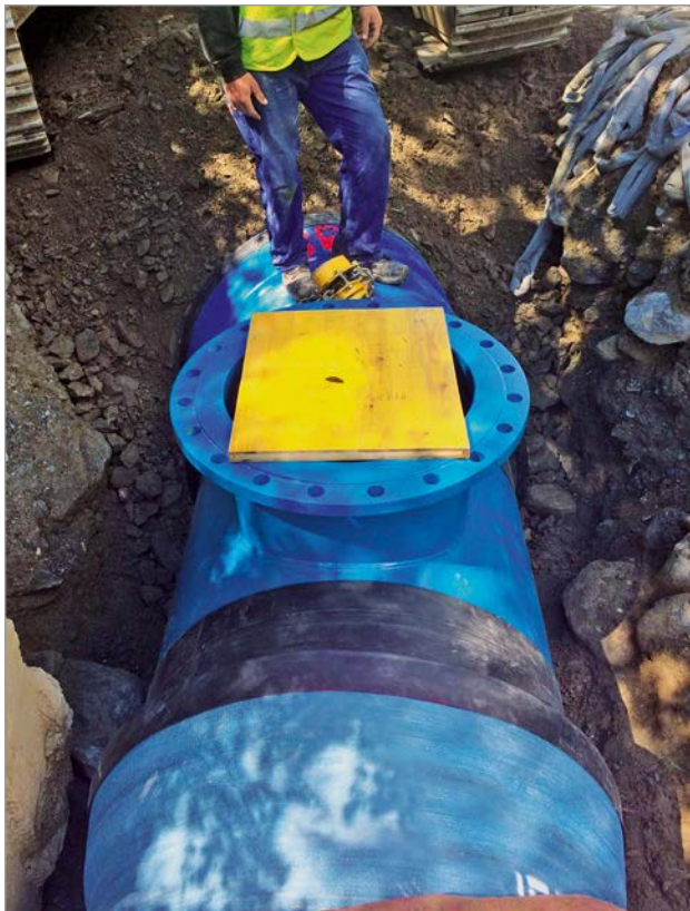
Figure 9: One of three manholes along the route of the power plant pipeline
