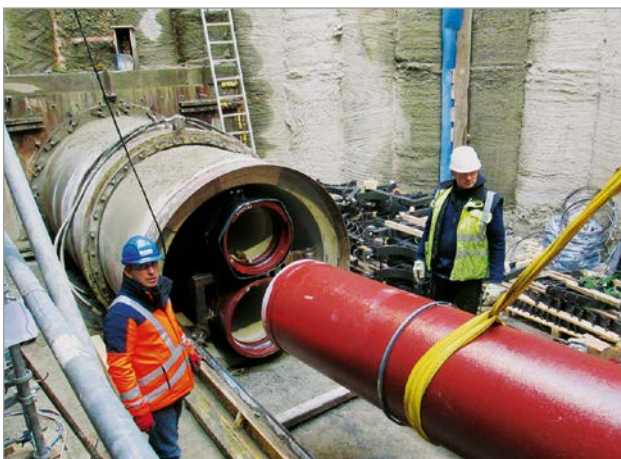
Figure 1: Installation of a DN 600 ductile iron pipe (the lower of the two) with a BLS® restrained push-in joint
