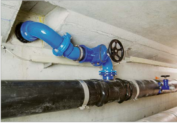
Figure 10: DN 125 branch pipeline to the hydrant recesses in the casing pipe (at the front in the picture) and flushing fitting with tapping saddle on the main pipeline (in the background)
