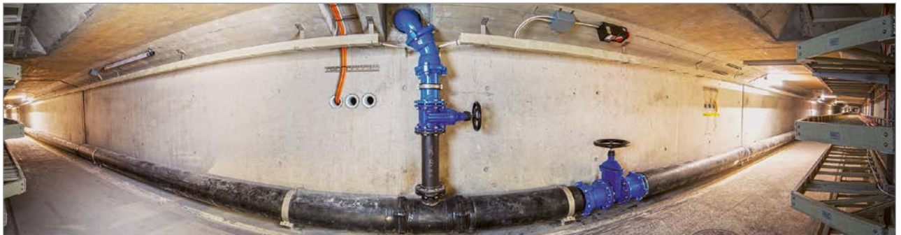
Figure 4: Panoramic view of the extinguishing water pipeline in the service conduit with side branch and section shutoff valve
