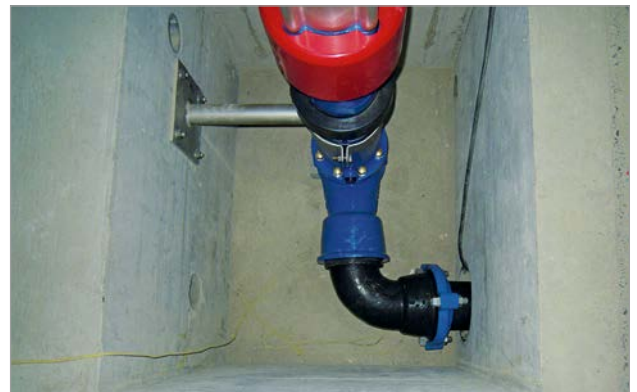
Figure 12: Hydrant recess with connection of the VARIO 2.0 hydrant lower part to the DN 125 branch pipeline
