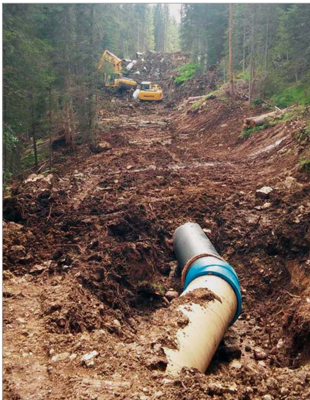
Figure 6: Construction on the unstable slope
