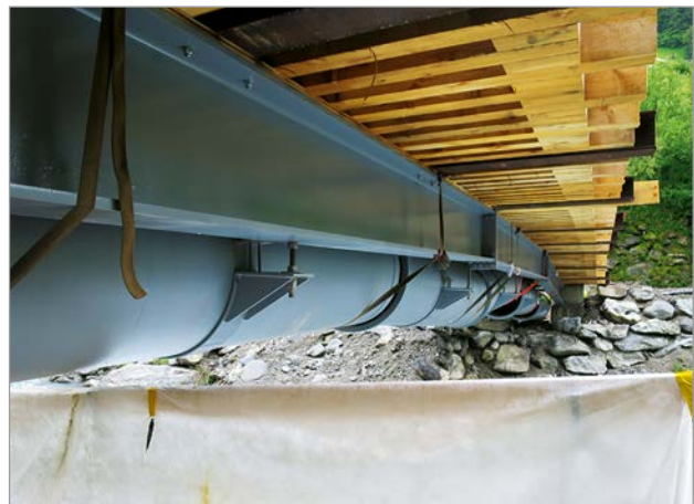
Figure 8: A view under the footbridge with the curved steel girders – the ductile iron pipes follow the contour of the curve
