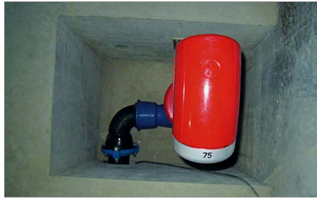
Figure 13: Tight space conditions for installing the hydrants
