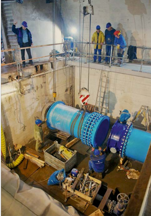
Figure 3: The DN 1200 flanged spigot and the DN 1200 dismantling joint are made ready as a single unit for assembly with the DN 1200 butterfly valve
