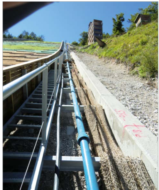
Figure 3: Ductile iron pipes with restrained VRS®-T push-in joints are part of the snow-making equipment of the Planica ski-jumping hill
