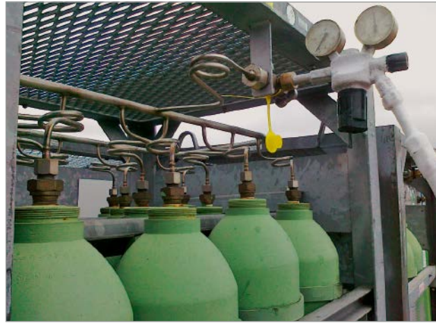
Figure 12: Bundle of cylinders as the source of CO 2
