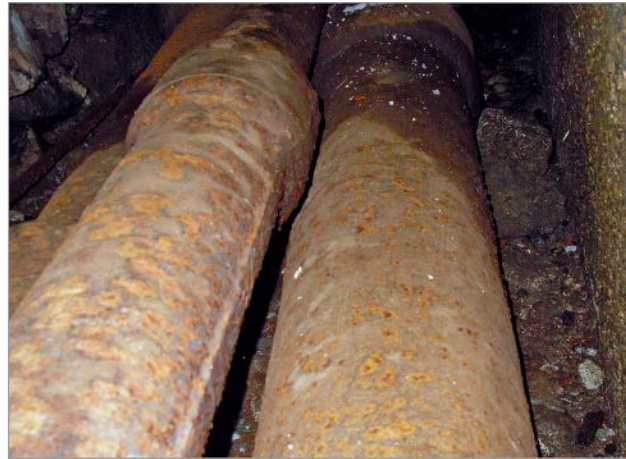
Figure 2: Cast iron piping in operation for the fountains of the UNESCO World Heritage "Wilhelmshöhe" mountain park in the Octagon beneath the Hercules statue [3]
