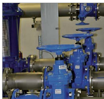
Figure 1: DN 150, PN 16 gate valves with DN 150, PN 16 nozzle check valves installed upstream
