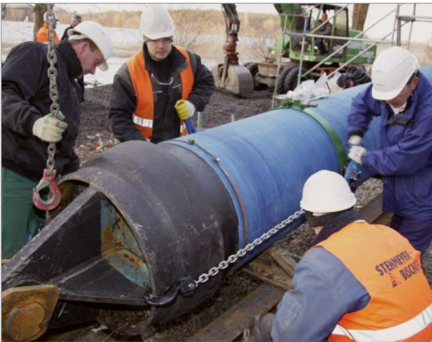
Figure 9: Directional drilling project on the River Havel in Berlin [12] – DN 700 ductile iron pipes – assembling the traction head – single pipe process
