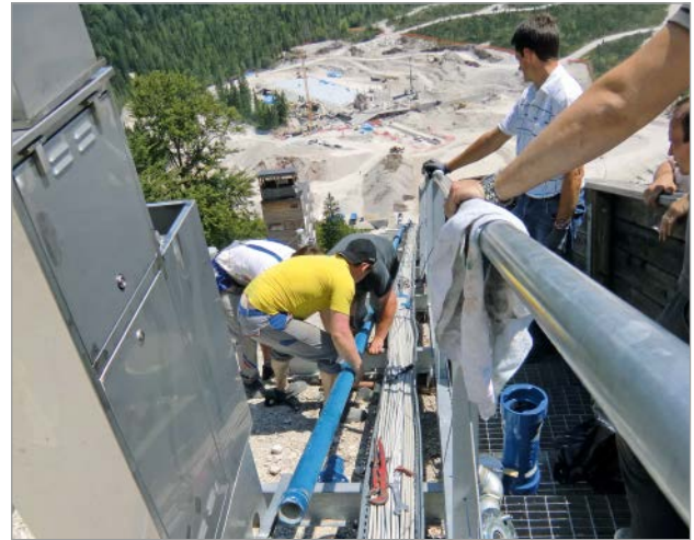
Figure 2: DN 80 ductile iron pipes – pipeline construction in the area of the starting position
