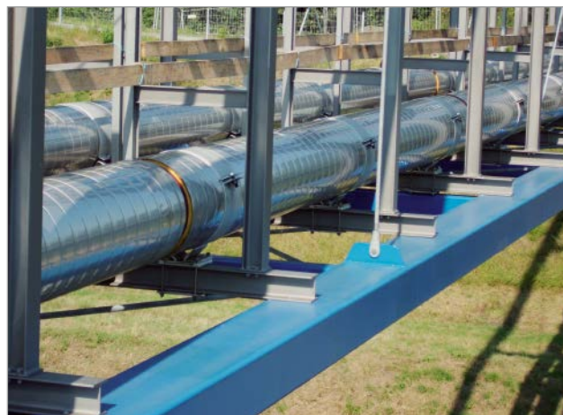
Figure 4: Exposed pipeline with folded spiral-seam outer tubing in stainless steel
