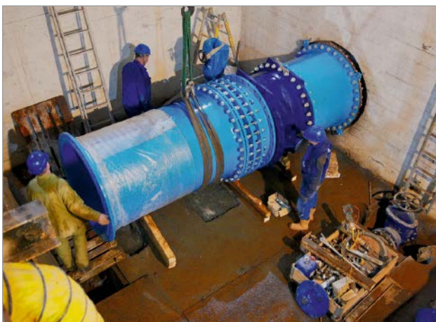
Figure 4: Both flanges of the DN 1200, PN 10 butterfly valve are connected to the existing pipeline components
