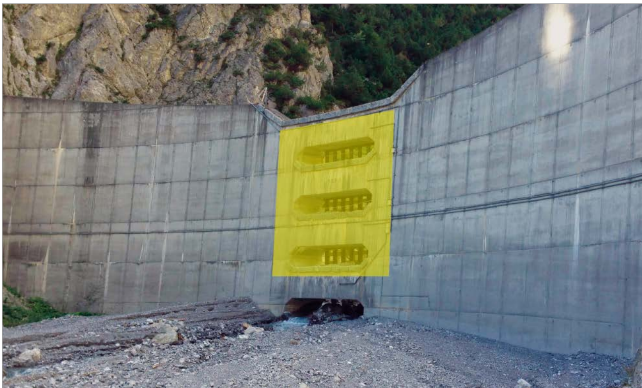
Figure 1: Arch dam on the Schnanner Bach – the three openings marked in yellow are each fitted with an inflatable weir system
