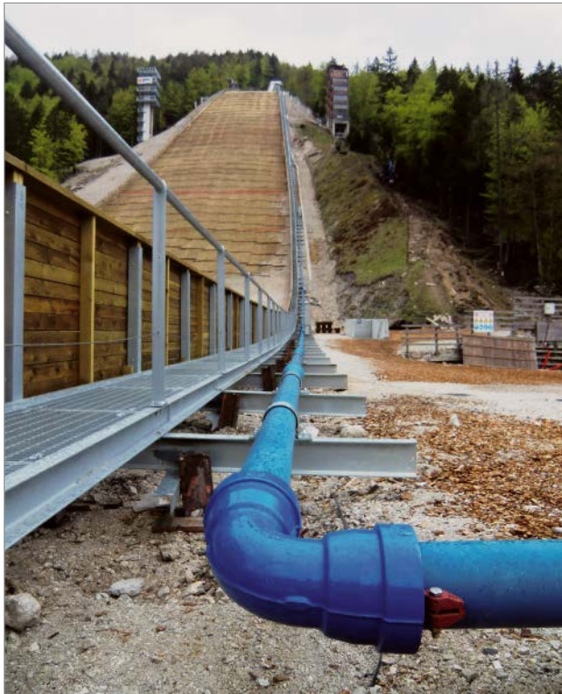
Figure 1: 90° bends incorporated in the restrained design VRS®-T DN 125 ductile iron pipeline in the run-out area of the ski-jumping hill
