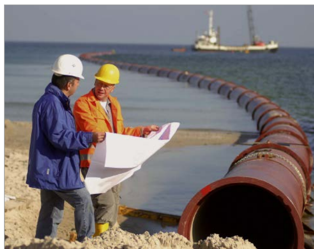
Figure 6: Planning and laying of a sea outfall pipe at Binz auf Rügen [9]
