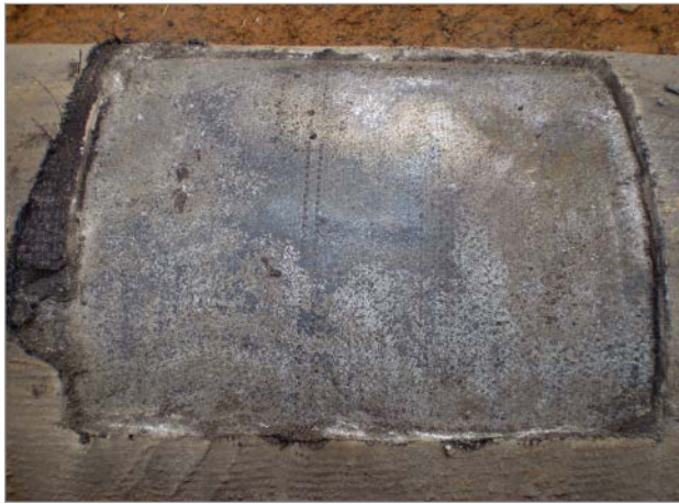
Figure 10: DN 400 ductile iron pipe installed in 1985 – cement mortar coating with epoxy bonding layer and zinc coating – exposed for checking in 2010: no visible corrosion attack [13]
