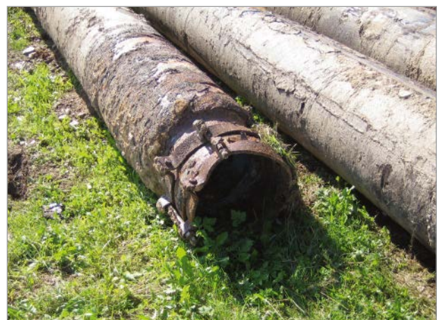
Figure 5: DN 350 steel pipes with handmade jointing elements removed from the old pipeline
