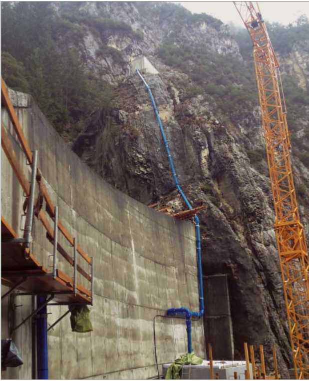
Figure 3: Ductile iron pipeline from the high-level tank to the barrier
