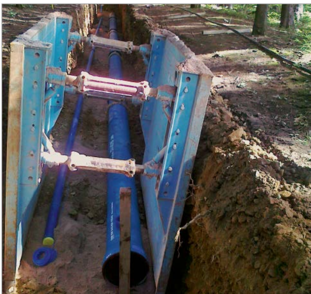
Figure 7: Installation of DN 400 ductile iron pipes with the help of shoring elements
