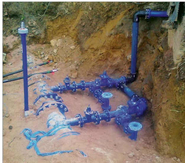
Figure 8: Laterally installed air valves
