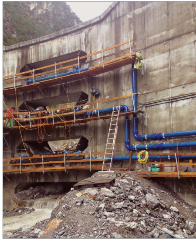
Figure 4: Ductile iron pipelines in the weir area
