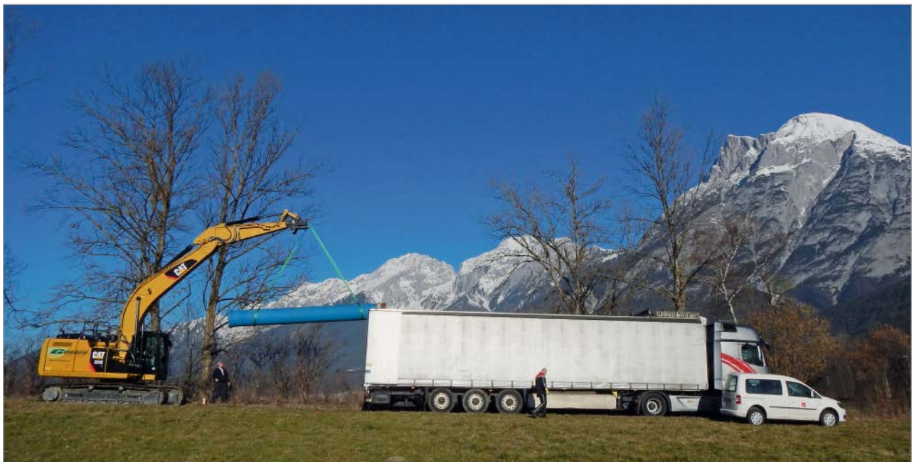
Figure 1: Delivery of ductile iron pipes for the turbine pipeline of the new hydropower station at Kanzingbach (Tyrol)
