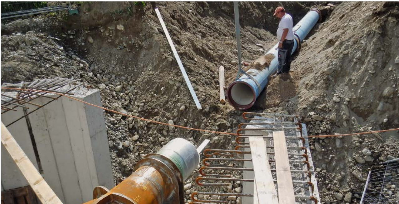
Figure 7: Laying the pipes with TYTON® push-in joints in front of the intake structure with a Y-pipe
