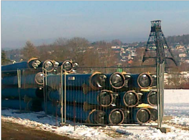
Figure 14: Construction site panorama with the old mining installations in the Western Ore Mountains
