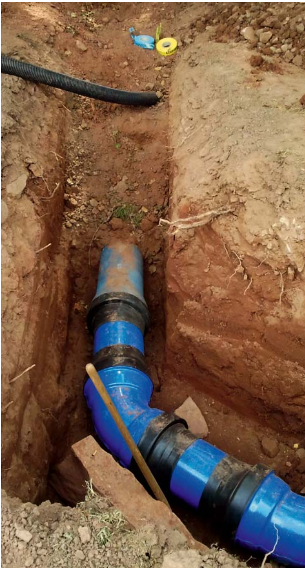
Fig. 5: Curve point at the transition from the BLS® push-in joint to the BRS® push-in joint
