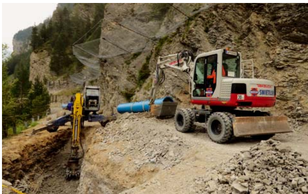
Fig. 8: Skilful use of a walking excavator with boring tool in steep terrain
