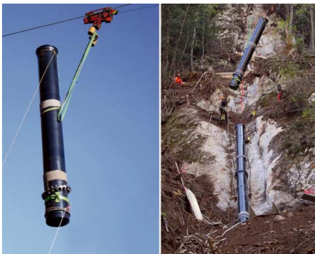
Fig. 5: Installation of vonRoll ECOPUR full-protection pipes with a site cableway in steep, inaccessible terrain
