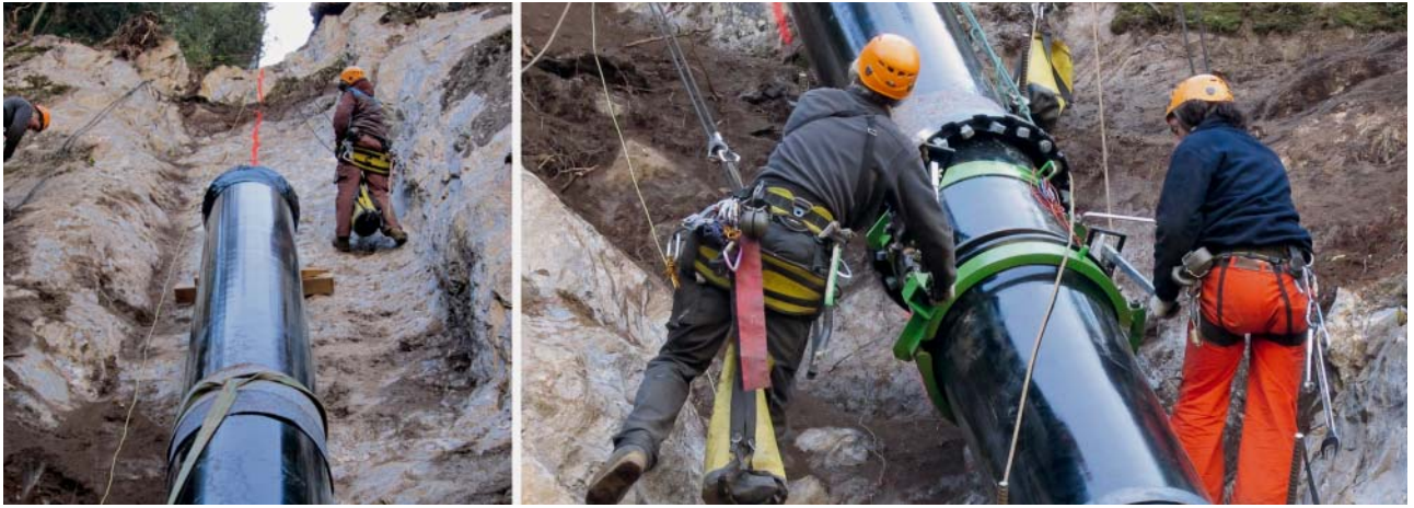
Fig. 4: Assembly of the ductile pipes above ground in the steep rock face
