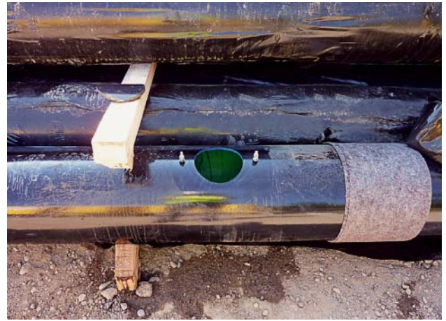
Fig. 3: Core drilling into a vonRoll ECOPUR pipe – the cutting edge is treated with a 2-component epoxy resin
