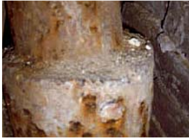
Fig. 2: The socket joint of an iron pipeline installed in the Octagon
