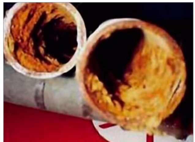
Fig. 2: Example of incrustations in pipelines
