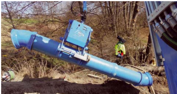
Fig. 5: Lifting a pipe section into the trench with the innovative system for ductile iron pipes
