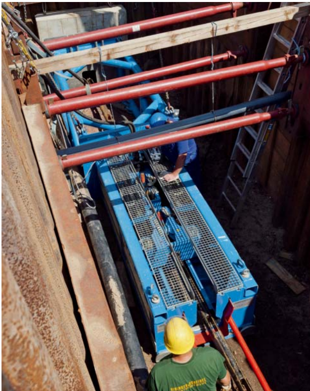
Fig. 5: GRUNDOBURST 1900G in the machine pit Source: BASF SE, Ludwigshafen
