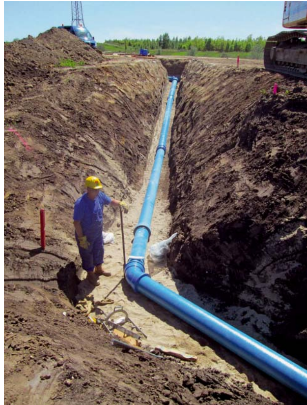
Fig. 3: Positive locking DN 250 ductile iron pipeline – concrete thrust blocks not necessary on bends
