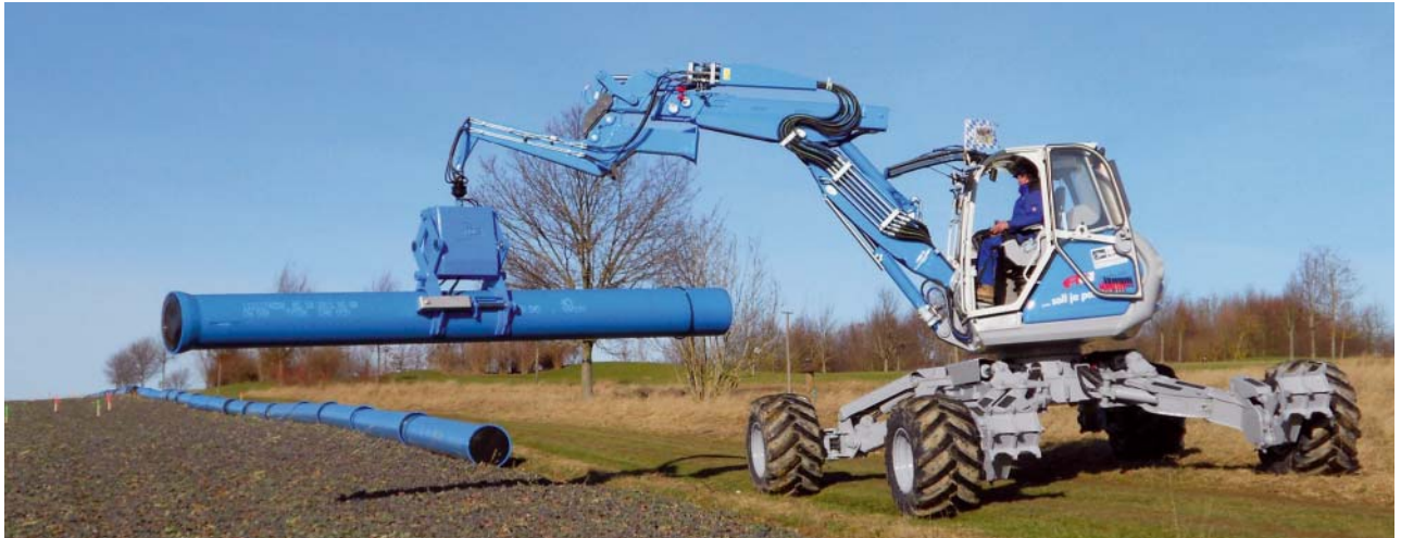
Fig. 2: Laying the ductile iron pipes along the route using a walking excavator
