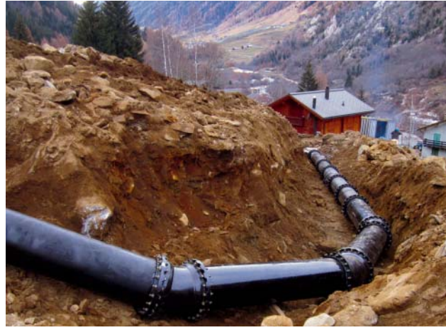
Fig. 3: vonRoll ECOPUR pipes with reinforced coating (PUR) to EN 545 [1], very resistant in rocky terrain, suitable for grain sizes 0-63 mm, largest size 100 mm, secured with vonRoll HYDROTIGHT thrust protection
