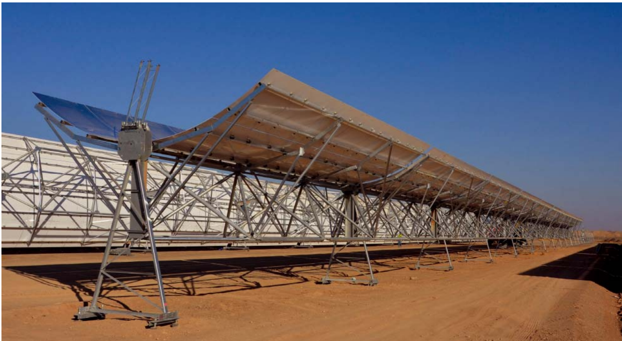
Fig. 1: CSP power station – parabolic reflector on the site of KaXu Solar One
