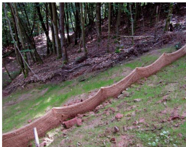
Fig. 8: Slope stabilisation of the route with jute mat prevents the topsoil from being washed away down the slope
