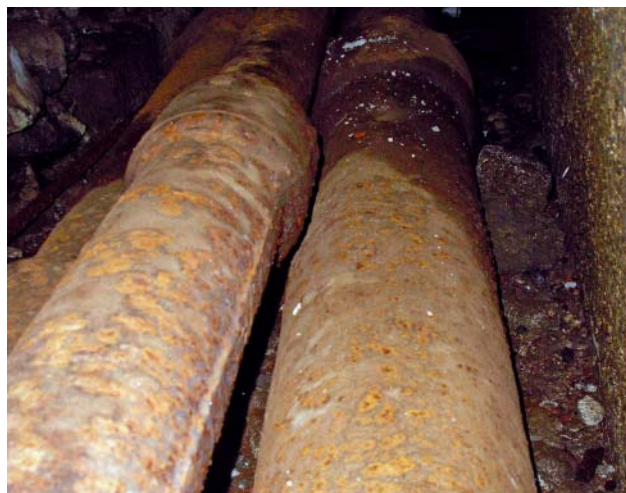
Fig. 3: Cast iron pipeline in operation in the Octagon UNESCO World Heritage Site – Bergpark Wilhelmshöhe
