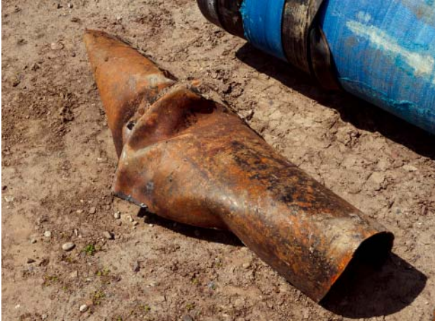
Fig. 9: Opened steel pipe (foreground) – slight scuff marks on the cement mortar coating of the ductile iron pipe (background)
