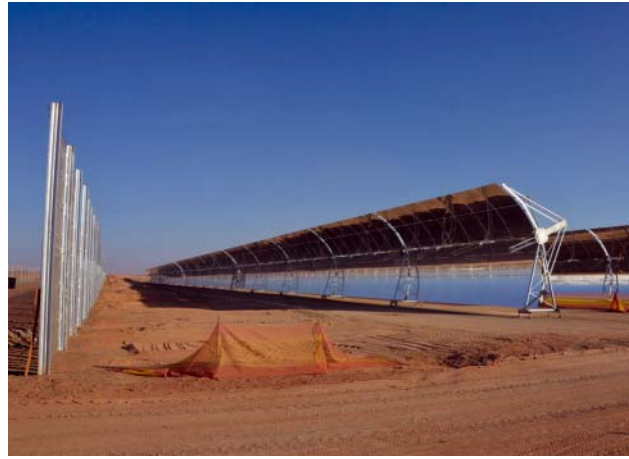
Fig. 5: 5 m high wind breaks protect the parabolic reflectors against high winds
