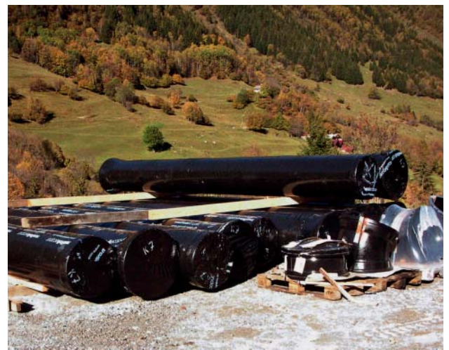
Fig. 6: Storage for ductile iron pipes and fittings
