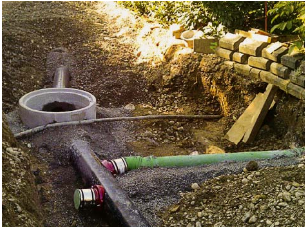
Fig. 2: Branch connection line to an existing building – connection by means of a tapping saddle and iron/plastic pipe transition sleeve
