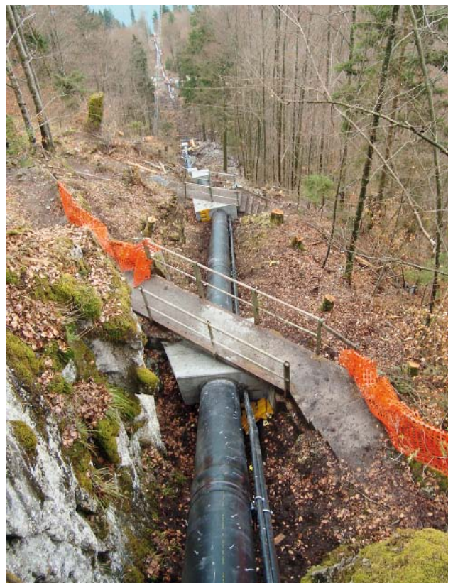
Fig. 6: Protective tubes for cables fixed to the ductile iron pipes with pipe clips
