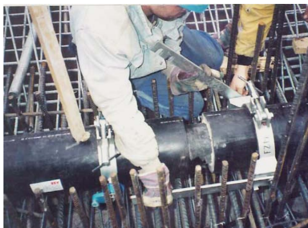
Fig. 12: Berlin's Tiergarten tunnel – Assembling WKG pipes within the reinforcement in the ceiling of the tunnel
