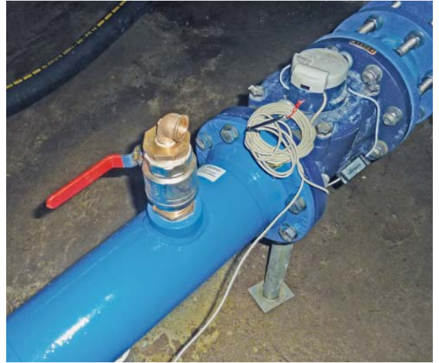
Fig. 1: Distributor 1 – internal measurement to monitor for pipe fractures: DN 150 welded-flange pipe with 2" connecting thread
