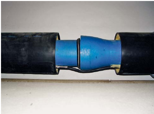
Fig. 14: Berlin Tegel airport – DN 125 WKG pipes installed in the tunnel with trace heating
