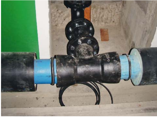
Fig. 13: Berlin Tegel airport – a branch pipe off the DN 125 WKG pipeline; installation in a trough in the tunnel
