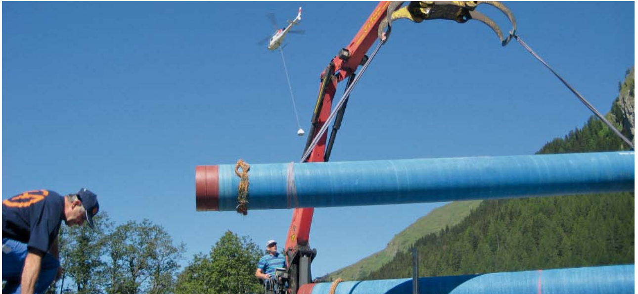
Fig. 8: The “Tambobach” penstock pipeline: on-site assistance by the excavator with the installation of the ductile iron pipes
