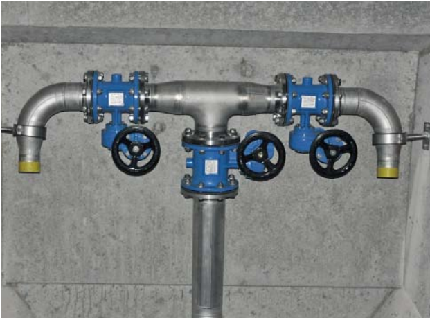
Fig. 12: Hydrant for supplying fire-fighting water
