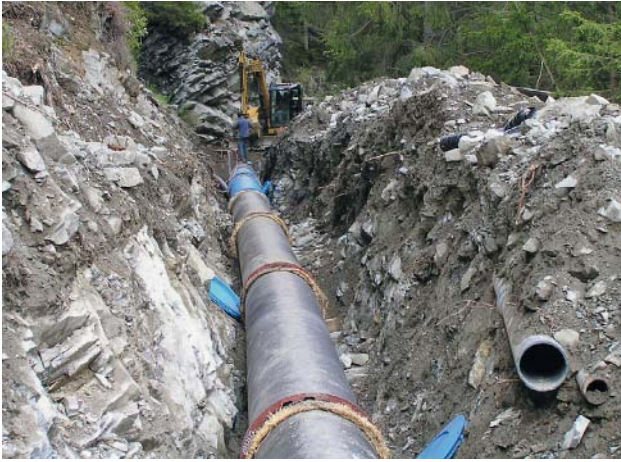
Fig. 8: The DN 600 ductile iron pressure pipeline in very rocky terrain
