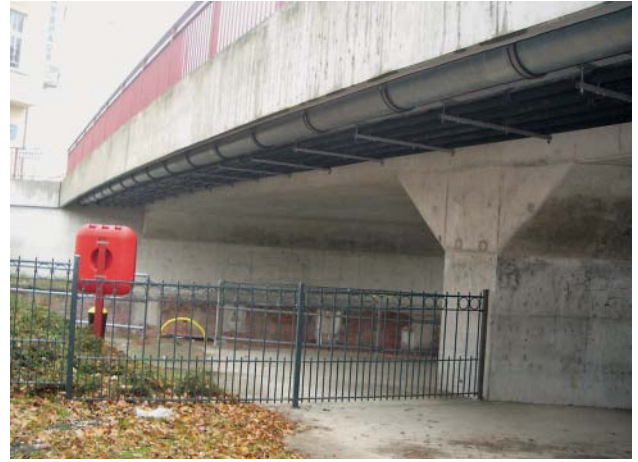
Fig. 21: The Rathenow lock: a WKG pipeline suspended below the road bridge behind a concrete skirt
