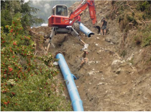
Fig. 1: Installing the ductile iron pipeline with the help of a walking excavator
