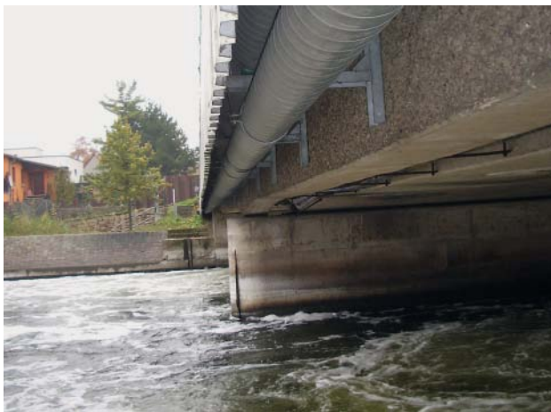
Fig. 20: The Brandenburg lock: a WKG drinking water pipeline suspended behind an outer skirt of trapezoidal profile metal panels
