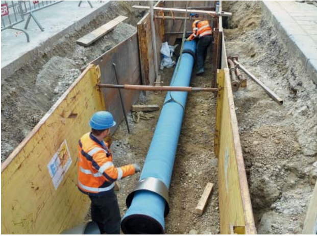
Fig. 4: A DN 400 cement mortar coated pipe with a BLS®/VRS®-T push-in joint in the installation pit
