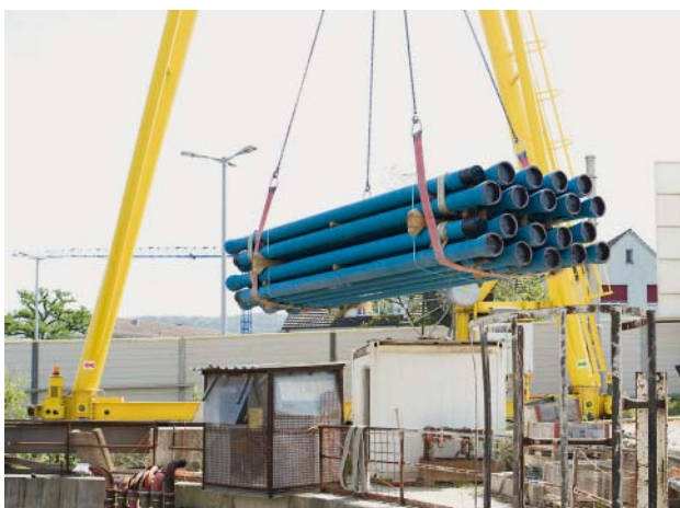
Fig. 8: Lifting the bundles of DN 200 pipes in via the existing launch shaft
