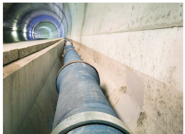
Fig. 11: Pipe supports in the utility channel
