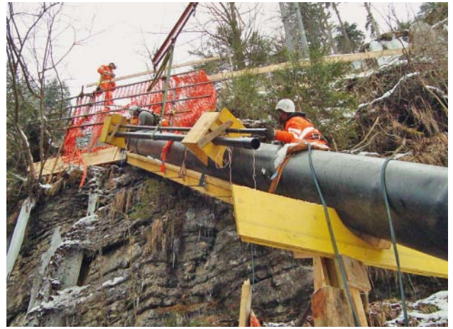
Fig. 5: The ductile iron pipes being installed in the region of the generator building, working from the top down
