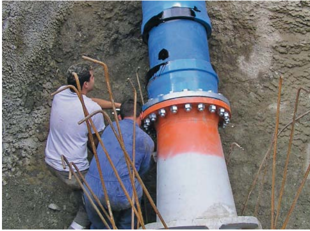
Fig. 11: Transition from a ductile iron pipe to the bifurcation pipe made with a flanged joint
