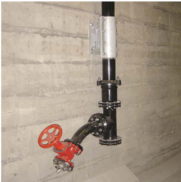
Fig. 14: Hydrant pipeline with temporary Storz fire hose connection
