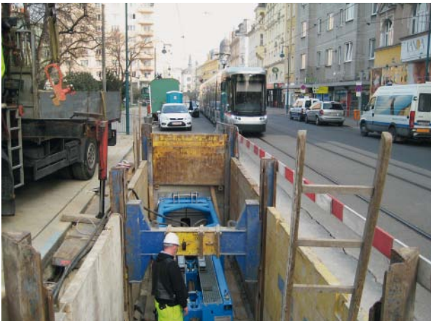
Fig. 3: A 1,900 kN tractive force traction rig made by the TRACTO-TECHNIK GmbH & Co. KG company being used for the first time in Austria.
