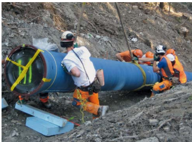
Fig. 5: The “Sagenbach” penstock pipeline: the DN 600 ductile iron pipes being assembled in difficult terrain
