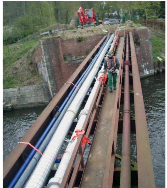
Fig. 17: A pipeline bridge for services in Potsdam – DN 200 WKG drinking water pipes with folded spiral-seam outer tubing
