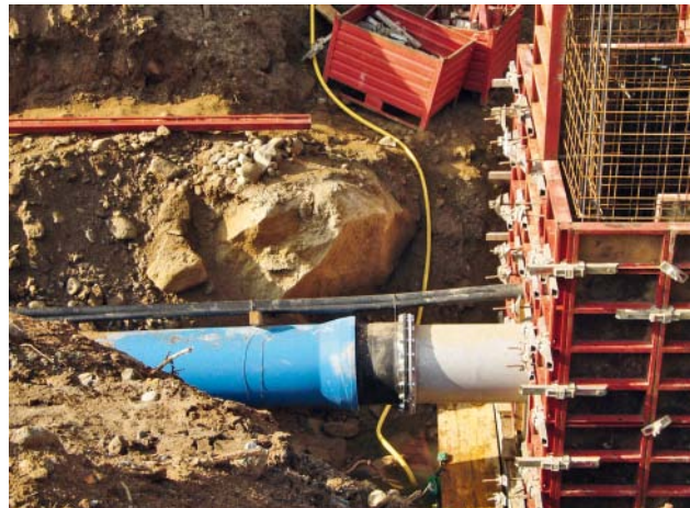
Fig. 4: The penstock pipeline connected to the de-sander by means of a flanged spigot
