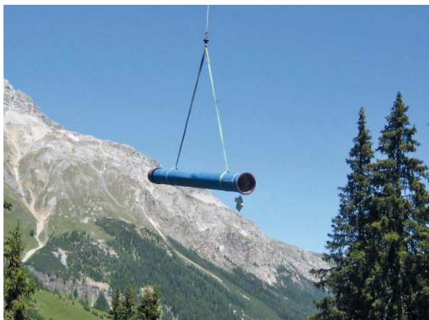
Fig. 7: The “Tambobach” penstock pipeline: a ductile iron pipe on the approach flight to the installation site
