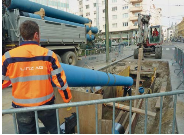
Fig. 6: Unloading a new DN 400 ductile iron pipe and lowering it into the pipe insertion pit
