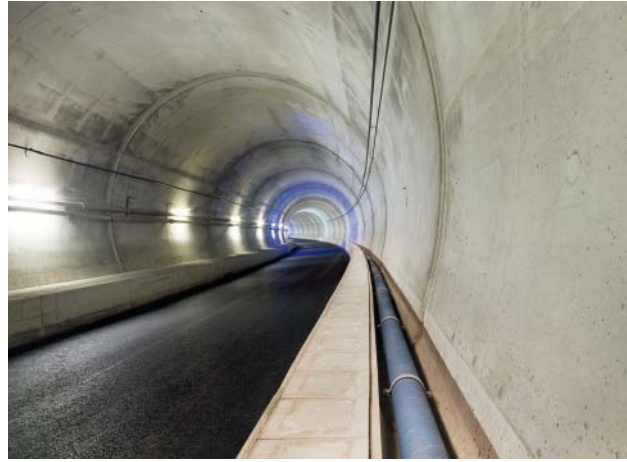
Fig. 13: Installed section of pipeline radiused through a curve – rapid transit trains will pass this point at 120 km/h
