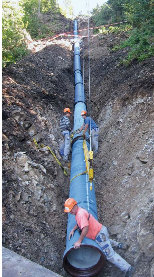
Fig. 12: The “Buoholzbach” penstock pipeline: looking along the route of the pipeline – ductile iron pipes with a cement mortar coating
