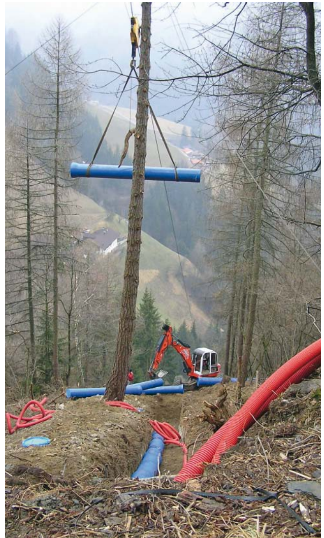
Fig. 7: The ductile iron pipes being brought in by a goods-carrying cable car
