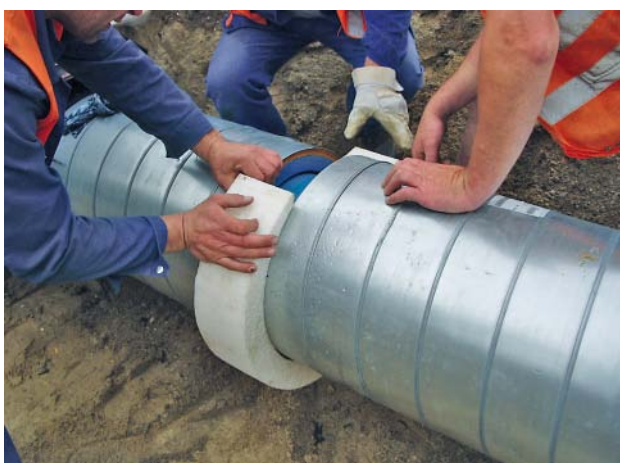
Fig. 8: Inserting the slit rings of foam material in the region of the socket joint
