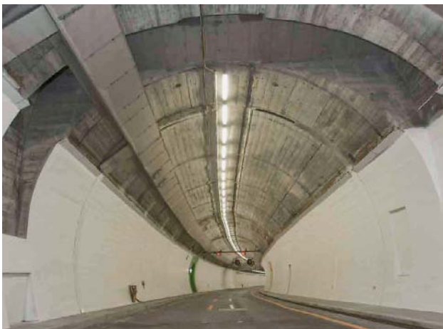
Fig. 2: An armoured door in the Sonnenberg tunnel
