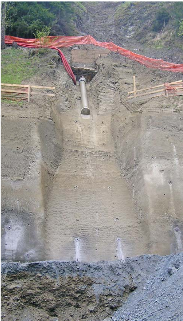
Fig. 9: The final ductile iron pipe before the connection to the turbine house
