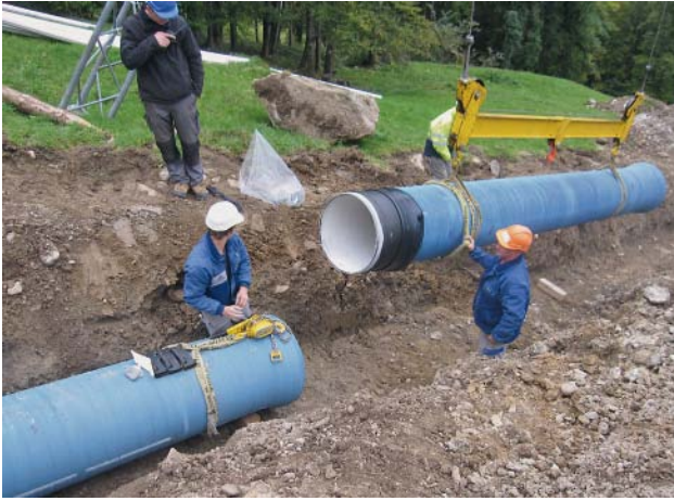
Fig. 11: The “Buoholzbach” penstock pipeline: Preparations completed for assembling a BLS® push-in joint
