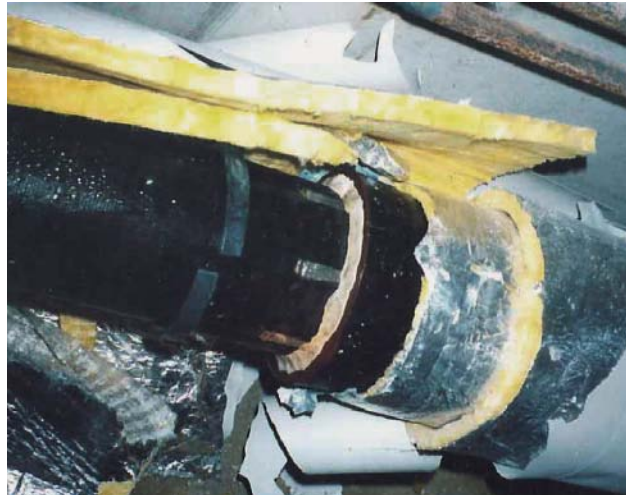
Fig. 3: A SIT® push-in joint in a section of pipe insulated by hand after being forced apart by exposure to frost
