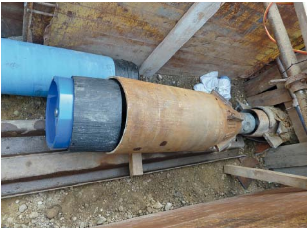
Fig. 5: The old grey cast iron pipeline having been burst, the passage was upsized to 610 mm at the same as the new DN 400 ductile iron pipes were pulled in
