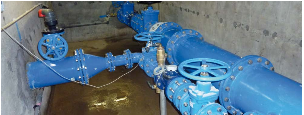
Fig. 2: Distributor 3 – new transfer point: passage through the wall by a DN 250 welded-flange pipe with a puddle flange and by a DN 80 flanged connecting pipe
