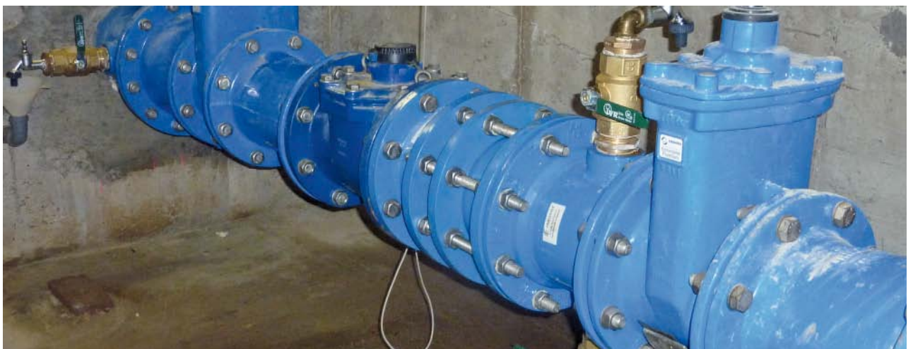
Fig. 3: Distributor 3 – internal measurement to monitor for pipe fractures: DN 100 welded-flange pipe with 2" connecting thread
