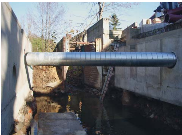
Fig. 15: Crossing over a receiving water in Neuzelle – DN 200 WKG pipes with folded spiral-seam outer tubing
