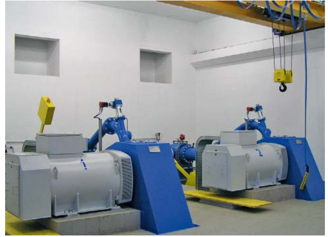
Fig. 12: From the bifurcation pipe, the driving water is distributed to two Pelton turbines
