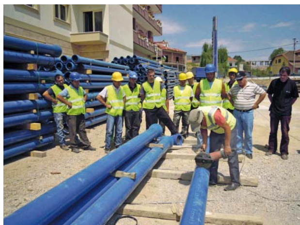
Fig. 3: The installation crews were given on-site instruction in Bilisht on all the subjects relevant to installation
