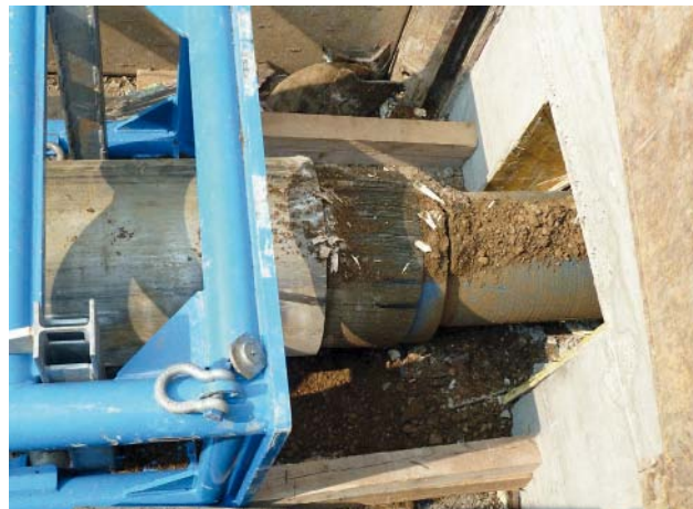
Fig. 7: The new DN 400, K 9, ductile iron pipeline arriving in the machinery pit
