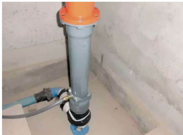
Fig. 4: Drainage facility for the closed hydrant through an angle connection for drainage
