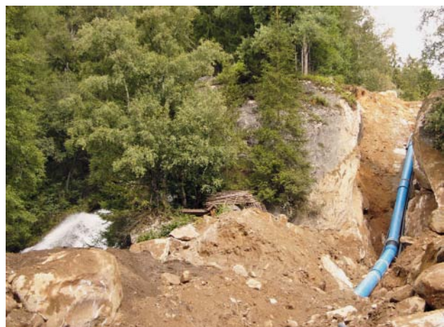
Fig. 5: The pressure pipeline runs through a wall of rock which has been blasted away
