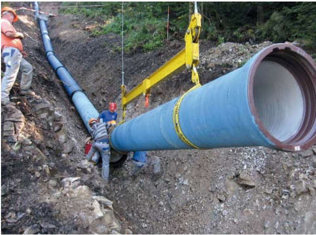
Fig. 13: The “Buoholzbach” penstock pipeline: open trench installation – the ductile iron pipes being installed with the help of the excavator
