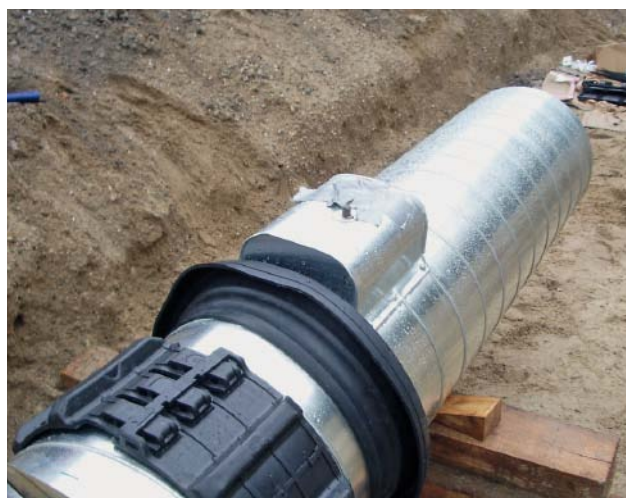
Fig. 5: A thermally insulated Hawlinger valve for air release on a WKG pipe
