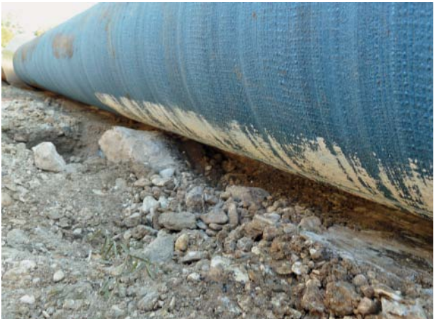
Fig. 7: The surface of the ZM-U coating under stress
