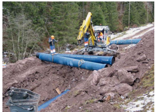
Fig. 10: The “Niedererbach” penstock pipeline: open trench installation – the DN 600, K 9, ductile iron pipes being installed with the help of the excavator
