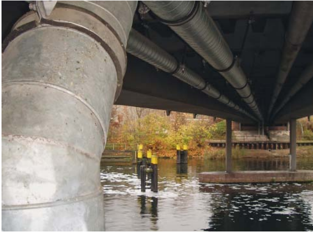
Fig. 19: The Wernsdorf lock: twin WKG pipelines suspended below the road bridge
