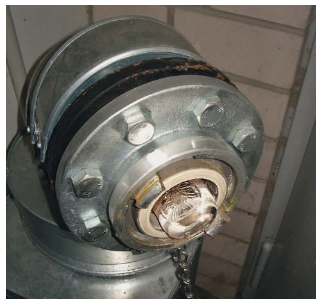
Fig. 2: Ice in a frozen hydrant
