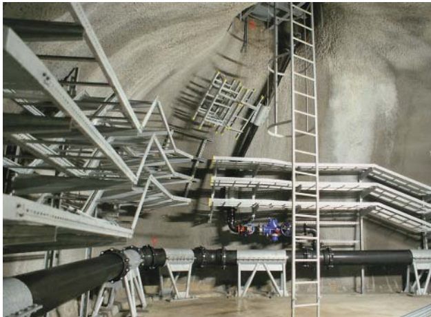
Fig. 7: Connecting pipeline between utility gallery and cross-passage in the Reussport tunnel
