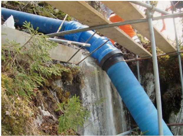
Fig. 4: A fixed point on the pipeline
