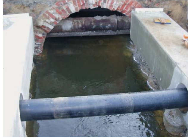
Fig. 16: Crossing over a receiving water on the Bahnhofstraße in Beeskow – WKG pipes with polyethylene outer tubing
