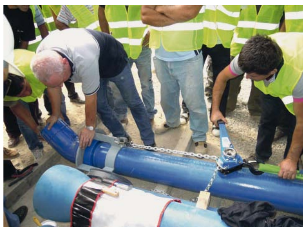
Fig. 4: Training in pulling a ductile iron bend onto the spigot end of a ductile iron pipe
