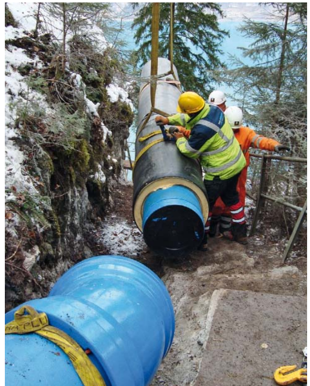
Fig. 3: Used a restrained fitting in the form of a bend to deflect a ductile iron pipeline angularly to adapt it to the route
