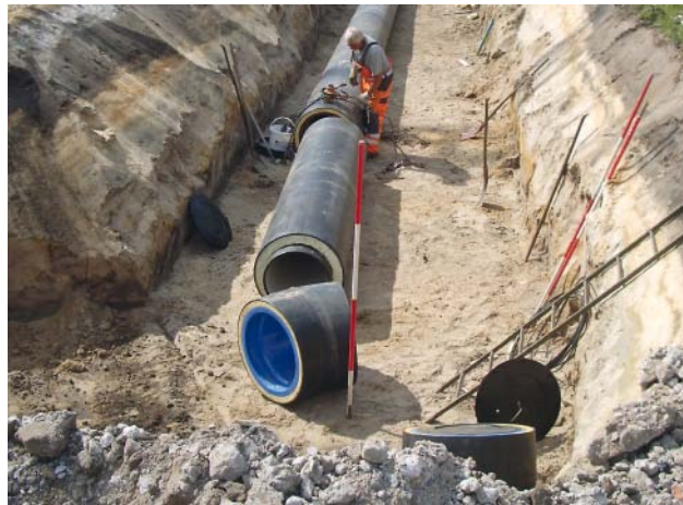
Fig. 11: The Sedlitz project – Installing the DN 500 WKG pipes in the open pipeline trench
