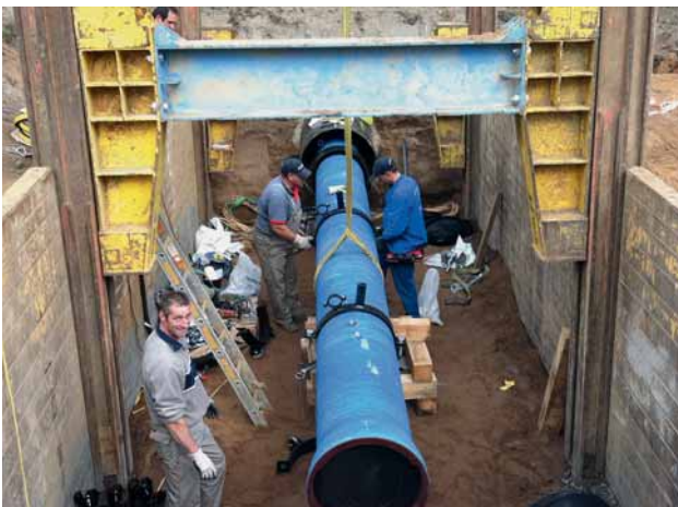
Fig. 4: Fitting the skids for sliding to a DN 500 ductile iron pipe – in preparation for the pulling-in
