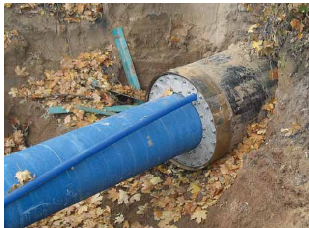
Fig. 7: The annular gap sealed off at the end of the steel protective casing tube – the annular gap was not filled.
