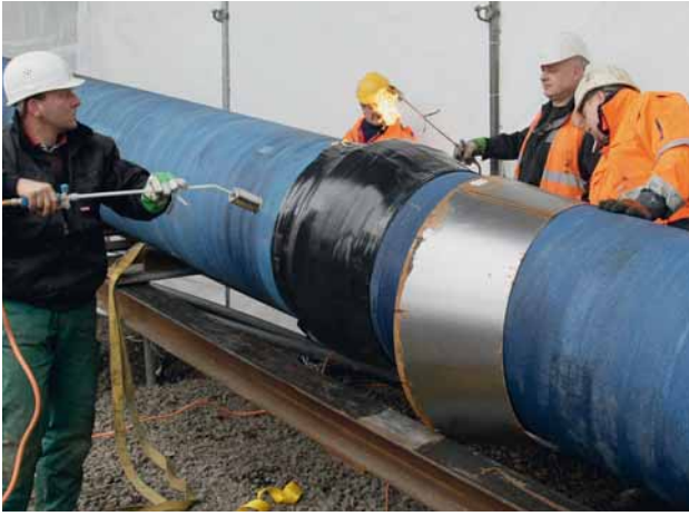
Fig. 7: The steel assembly ramp – A shrink-on sleeve and protective cone being fitted
