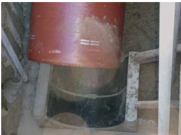
Fig. 7: Installing the DN 800 ductile iron pipes – pipes supported on neoprene-lined concrete cradles
