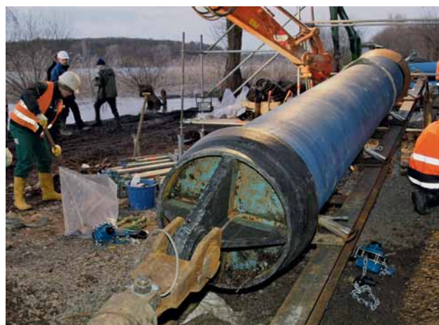
Fig. 6: Pipe-by-pipe assembly – the first DN 700 ductile iron pipe on the assembly ramp
