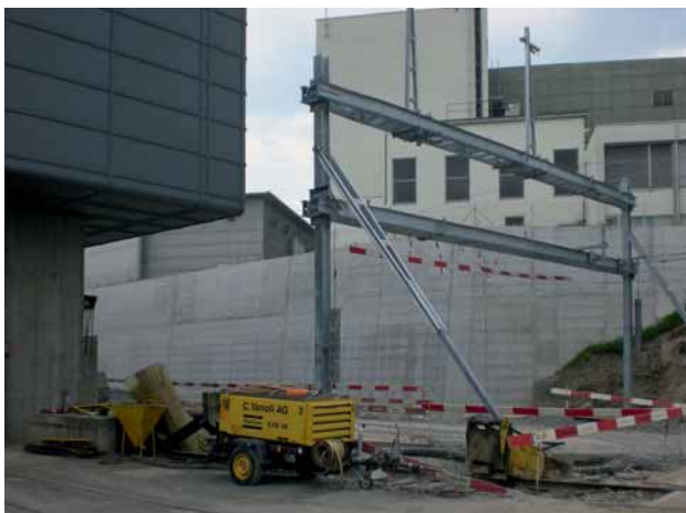
Fig. 13: New Swiss Federal Railways overhead lines: the piles for the mast and anchorage footings are loaded in tension and compression and the horizontal forces are coupled with the moments and are applied to the top of the footings.
