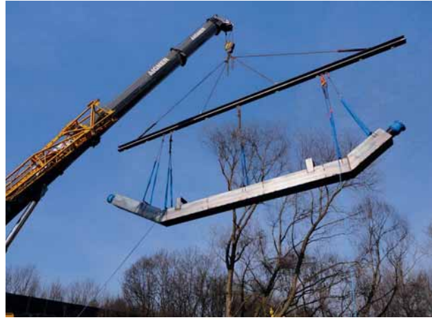
Fig. 6: The culvert pipelines were lowered into place by heavy cranes to cross some smaller waterways
