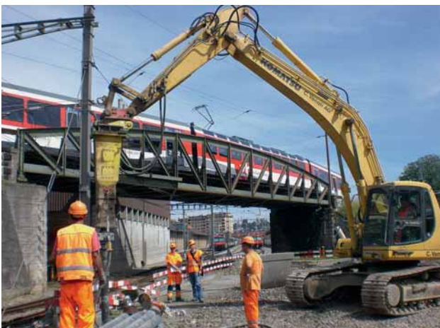
Fig. 8: Thanks to the light and compact driving equipment, the ductile iron piles were installed directly by the existing tracks and overhead lines, with restricted headroom, while normal railway services continued.
