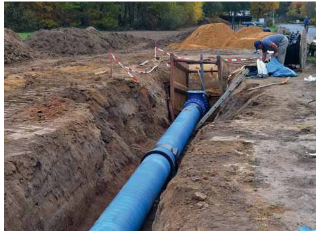
Fig. 6: DN 500 restrained ductile iron pipes with a cement mortar coating and shrink sleeves plus protective cones at the socket joints
