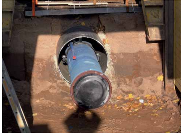
Fig. 5: A DN 500 ductile iron pipe pulled into the DN 900 steel protective casing tube
