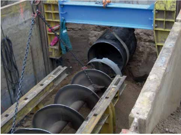
Fig. 2: Removing the soil from an installed DN 900 protective casing tube with a feed auger
