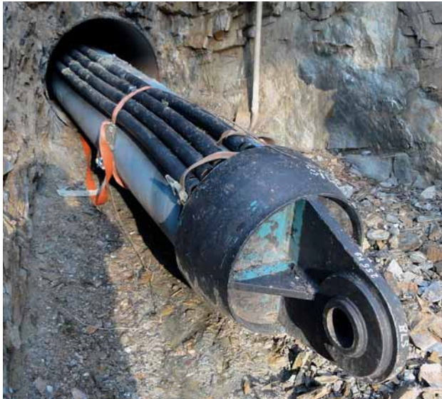
Fig. 8: At the tunnel exit: the traction head with ductile iron pipes hitched on with four empty pipes riding on them
