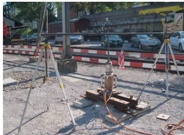
Fig. 11: A tension pile being tested: in the tensile test, the test pile operating by skin friction achieved the requisite load-bearing capacity with a safety factor of 3.5.
