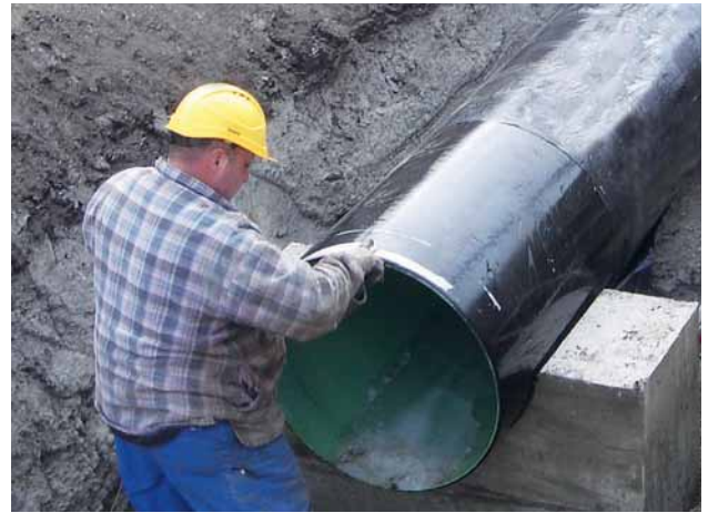
Fig. 7: Fitting vonRollgeocopur ductile iron pipes to a cradle of in-situ concrete at very low temperatures
