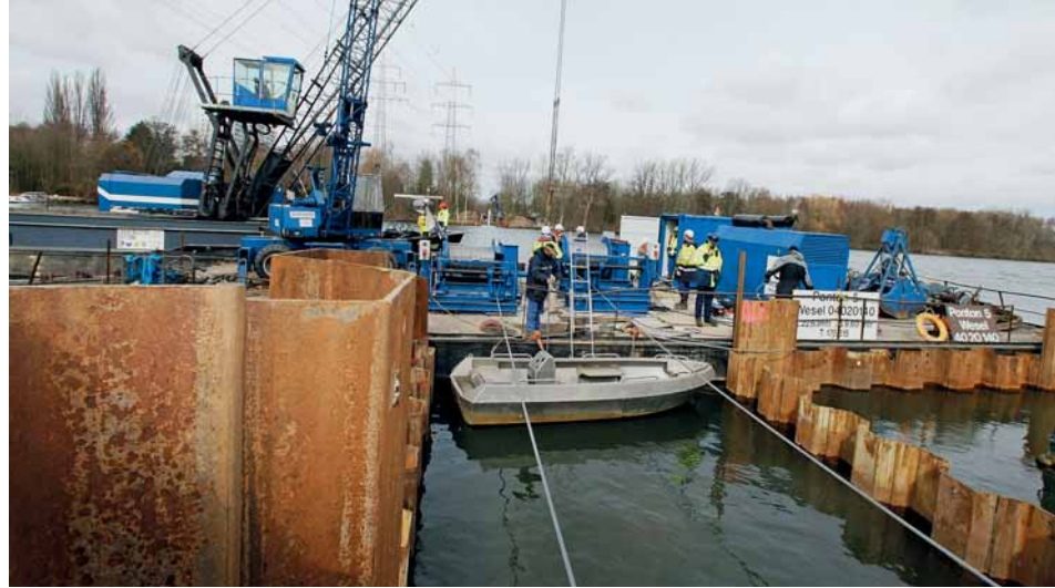
Fig. 11: Looking from the direction-changing frame over the cable winches to the left bank of the Main
