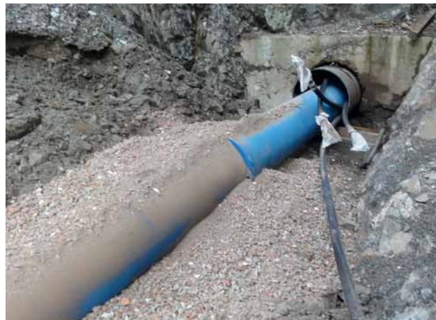
Fig. 6: The launch pit – an inserted steel tube with ductile iron pipes pulled in
