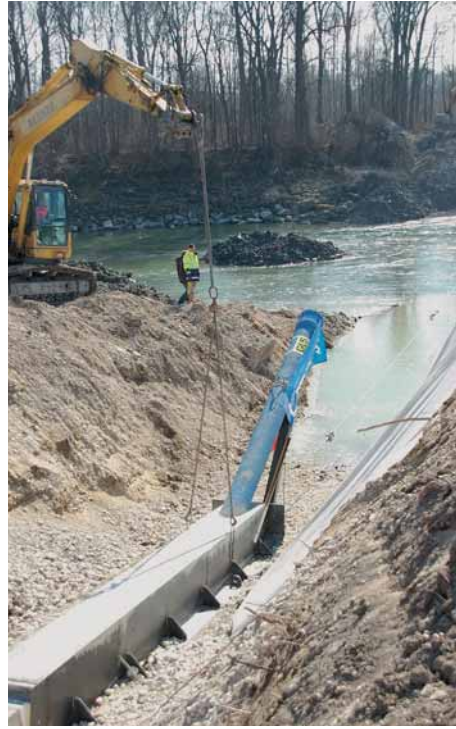
Fig. 1 (on the left): The DN 400 culvert pipeline before being pulled in – ductile iron pipes encased in concrete
