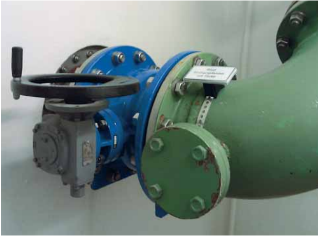
Fig. 1: Settling chamber outlet
