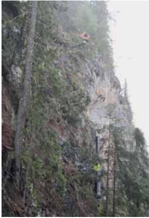
Fig. 7: Project 3 – The Furkelbach power station in South Tyrol: pipes being brought in by cable car
