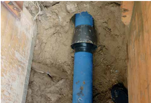
Fig. 7: Protection for the restrained push-in joint – a rubber collar and a sheet-metal cone
