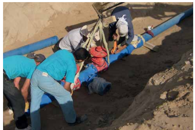
Fig. 4: Connection of ductile iron pipes, isolating gate valves and take-offs to underground hydrants
