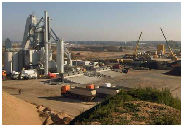
Fig. 2: A mobile concrete mixing plant on the apron of the new Terminal 3 soon to be built
