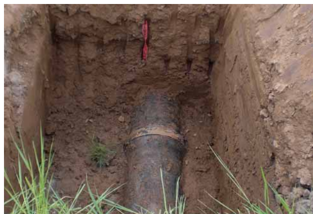
Fig 1: Project 1: Test dig – Heilbronn, Böllinger Höfe district, Wannenäckerstrasse – DN 400 ductile iron pipe, year of installation 1985
