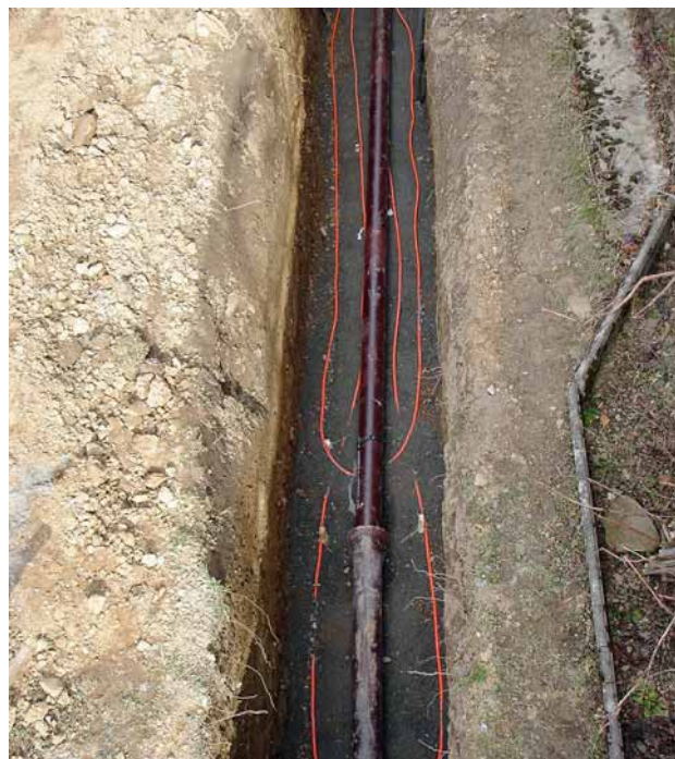
Fig. 2: DN 125 sewage pipeline of geopur type pipes. Plastic coated copper tubes for the refrigerant circuit are laid in the bedding
