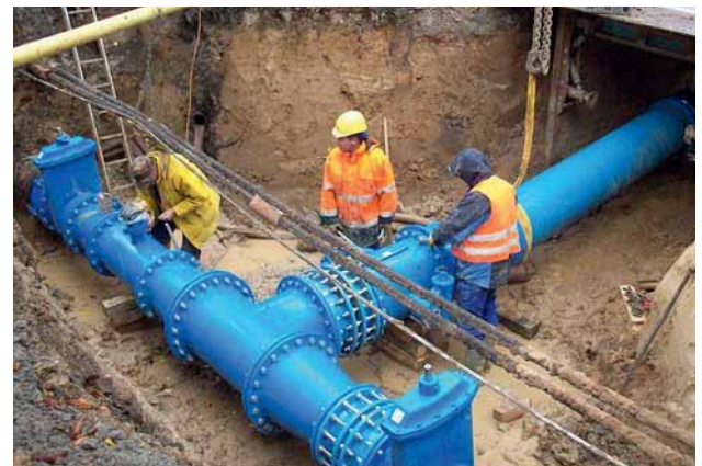
Fig. 4: Connecting the DN 500 ductile iron pipeline into the DN 800 pipeline, also of ductile iron
