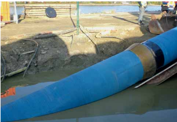
Fig. 9: Pulling-in of the pipes; the push-in joint is protected by shrink-on material and a sheet-metal cone slid over the top
