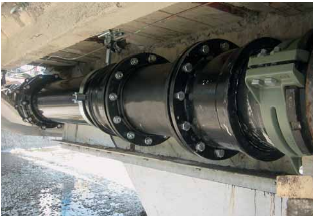
Fig. 8: Connection of the ecopur pipes to the existing screwed socketed pipeline on the city of Lucerne side
