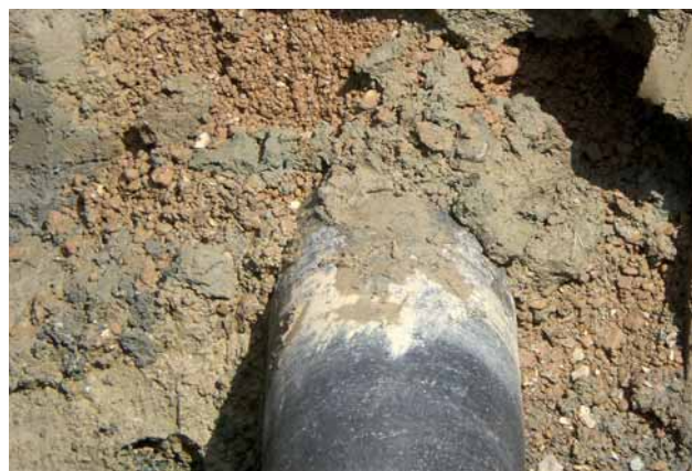
Fig. 9 Project 3: DN 300 ductile iron pipe – Soil in region of bottom of pipe slightly aggressive gravel, pipe embedded in highly aggressive soil at the sides and top, ground water present
