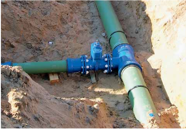
Fig. 3: A pipeline for fire-extinguishing water of DN 300 ductile iron pipes with a DN 150 branch for connecting in a hydrant
