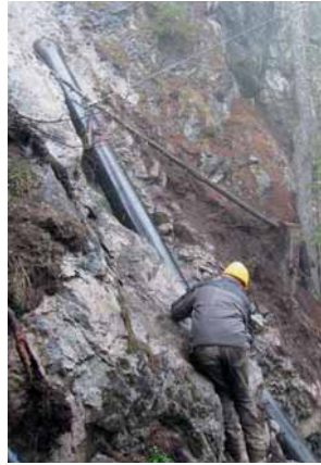
Fig. 8: Project 3 – The Furkelbach power station in South Tyrol: extreme conditions for pipe installation
