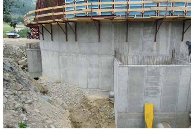
Fig. 2: Project 1 – The Vernagtsee power station in South Tyrol: the storage tank at 2,100 m above sea level
