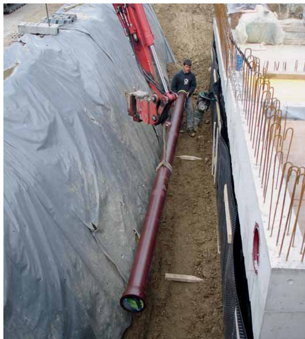
Fig. 1: Installation of the air pipeline for collecting geothermal heat – DN 200 geopur type ductile iron pipes
