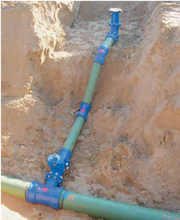
Fig. 4: Ductile iron pipes forming a DN 150 lateral for making a connection to a hydrant
