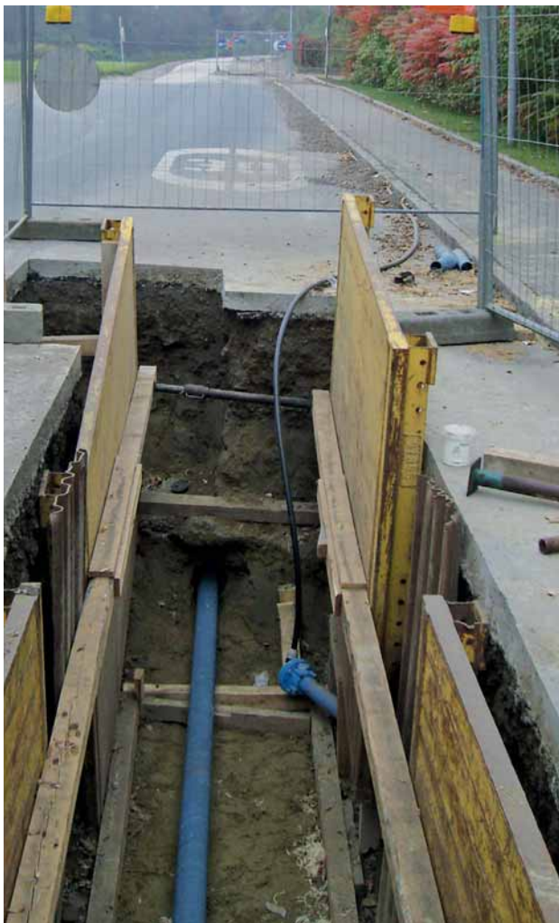
Fig. 4: A section showing a ductile iron pipe which has been pulled in
