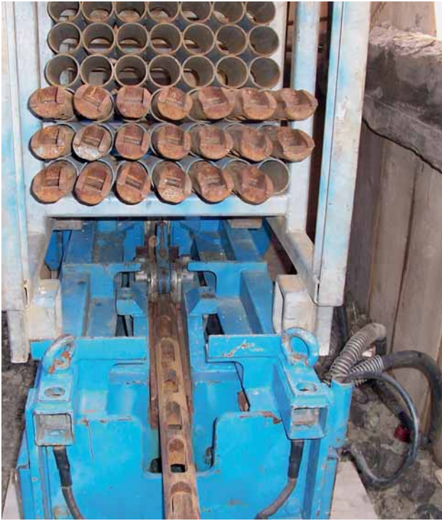
Fig. 1: The 400 G bursting rig
