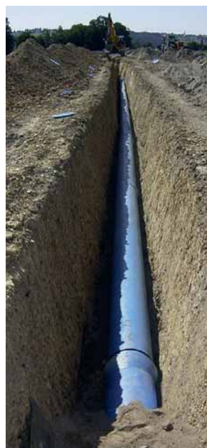
Fig. 4: Installation on the same route of DN 400 ductile iron drinking water pipes with BRS® restrained joints
