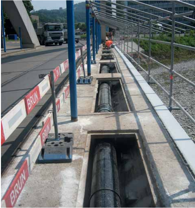
Fig 3: Opened access openings to the duct for the works pipeline, standard length of 3.40 m
