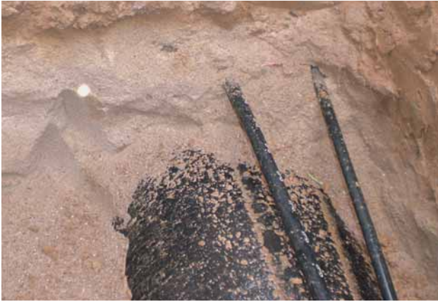
Fig. 6 Project 2 – DN 500 ductile iron pipe – Pipe embedded in not aggressive sand, native soil aggressive
