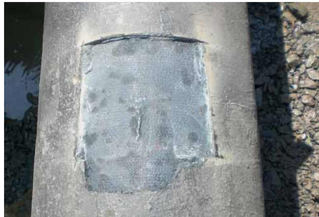
Fig. 8 Project 3: DN 300 ductile iron pipe - ZM-U with epoxy bonding layer, no zinc coating; no visible signs of corrosive attack
