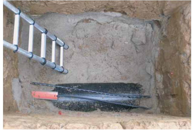
Fig. 4: Project 2: Test dig – Heilbronn, Böllinger Höfe district, lengthened part of Grundäckerstrasse – DN 500 ductile iron pipe, year of installation 1979
