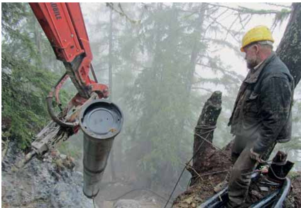
Fig. 9: Project 3 – The Furkelbach power station in South Tyrol: installation on a 65° slope
