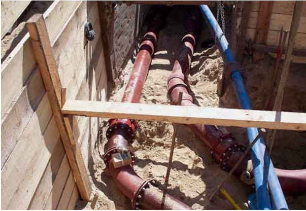
Fig. 6: The twin DN 250 pipelines as laid in the area of a bend
