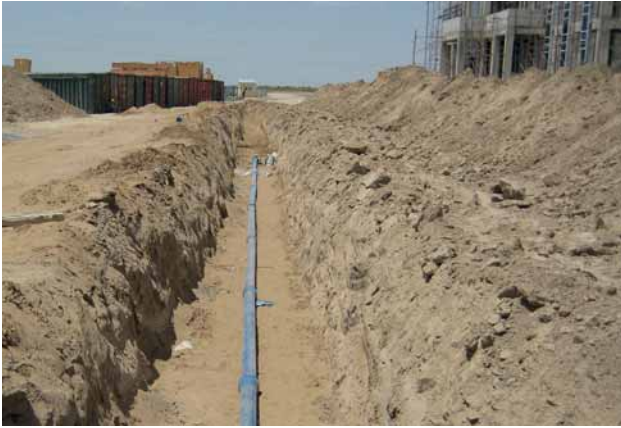
Fig. 5: A fire-fighting pipeline – a buried ring pipeline
