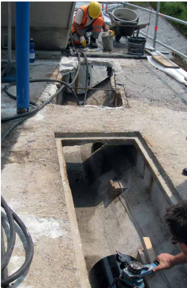
Fig. 4: The short access opening (length of 1.40 m) at the concrete abutment at the end of the bridge on the city of Lucerne side where the connection was made
