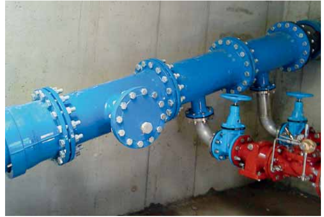
Fig. 10: Project 4 – The Holzerbach power station: valve manhole for several take-offs from the pipeline
