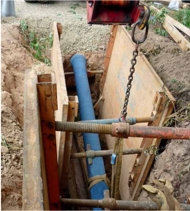
Fig. 6: A DN 200 ductile iron pipe being lowered into the pipe connection pit (starting pit)
