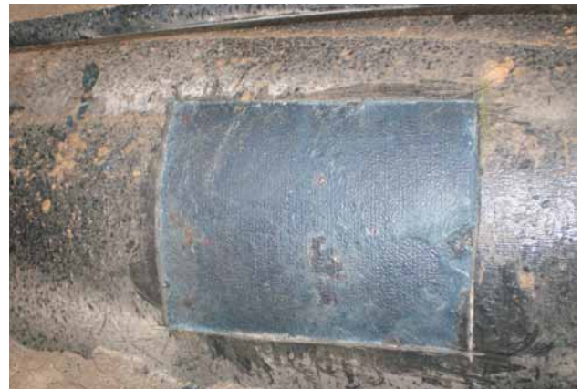
Fig. 5: Project 2 – DN 500 ductile iron pipe – ZM-U with epoxy bonding layer, no zinc coating; no visible signs of corrosive attack
