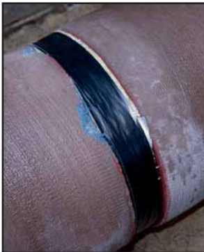
Fig. 5: A sealed gap in the region of the BLS® push-in joint of a ZMU-PLUS pipe
