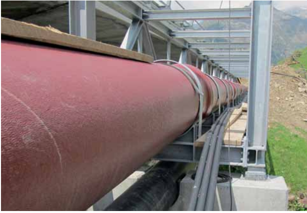
Fig. 4: Project 1 – The Vernagtsee power station in South Tyrol: the ductile iron penstock pipeline fastened in place with pipe clips
