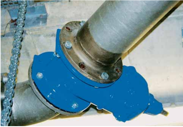
Fig. 3 Replacement of a DN 250 gate valve by a dismantling type butterfly valve in the course of inspection work by the Landeswasserversorgung Baden-Württemberg water supply utility
