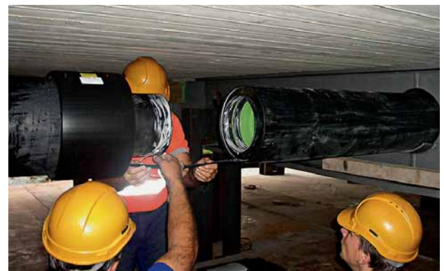
Fig. 4: The ecopur ductile iron pipe and its internal thrust resistance being prepared for the connection of the push-in joint.
