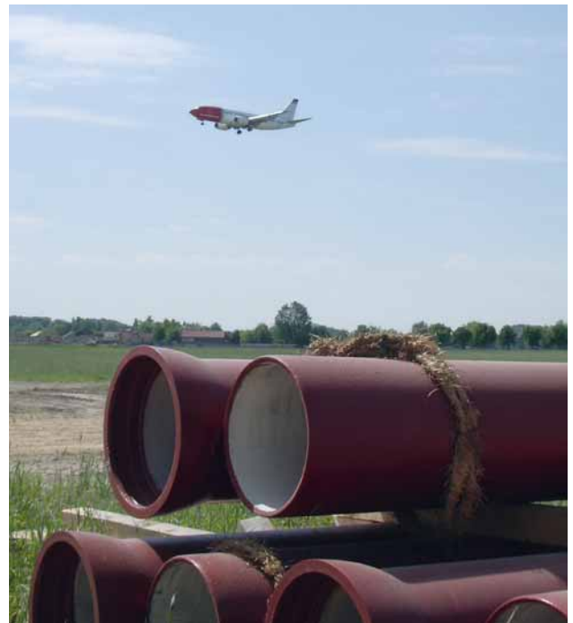
Fig. 1: Flying services are maintained in spite of the giant BBI construction site
