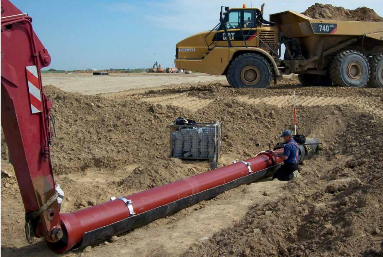
Fig. 9: BLS® socket-jointed DN 400 ductile iron sewer pipes being pushed into a run of casing tubes
