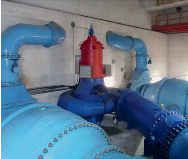
Fig. 2: The two needle valves and the turbine inside the dam (picture credit: Archive of Talsperrenbetrieb Sachsen-Anhalt)
