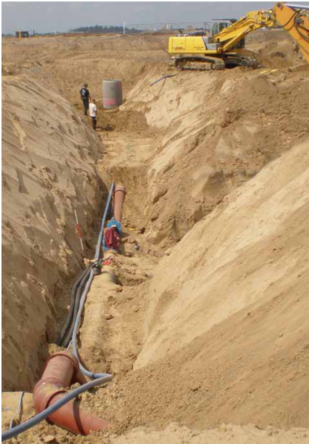
Fig. 8: Culverting under a structure to be erected later using DN 400 ductile pressure pipes
