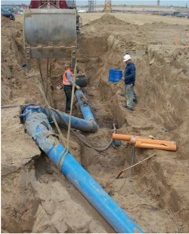
Fig. 7: A section of DN 300 pipeline retrospectively diverted sideways for a hydrant to be fitted
