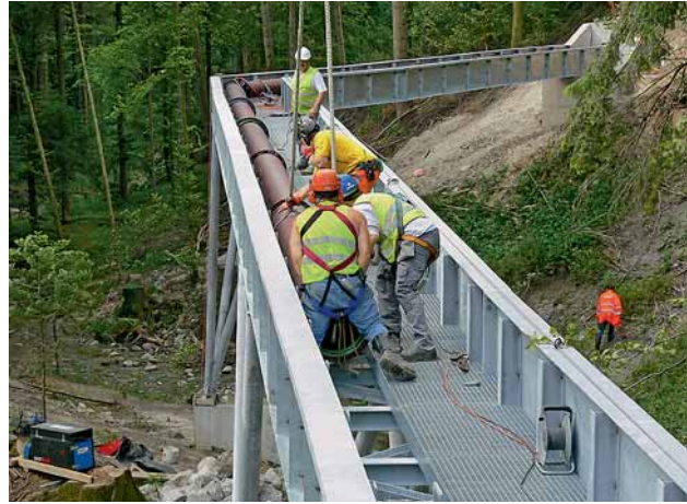
Fig. 6: The "Gämpi" walk-on sewer viaduct showing the DN 400 geopur pipes and their transport
