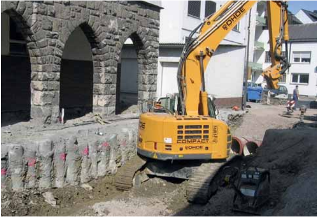
Fig. 4: The post-and-beam house shored up by a wall of secant bored piles
