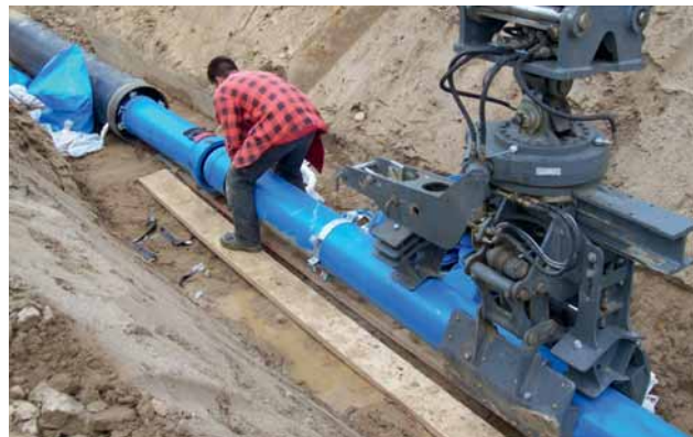
Fig. 6: A DN 300 ductile drinking water pipeline being connected and pushed in by special attachment
