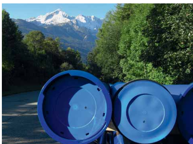
Fig. 1: Ductile iron pipes with BLS® push-in joints in the Wettersteingebirge mountain range – with the 2,628 m high Zugspitze in the background
