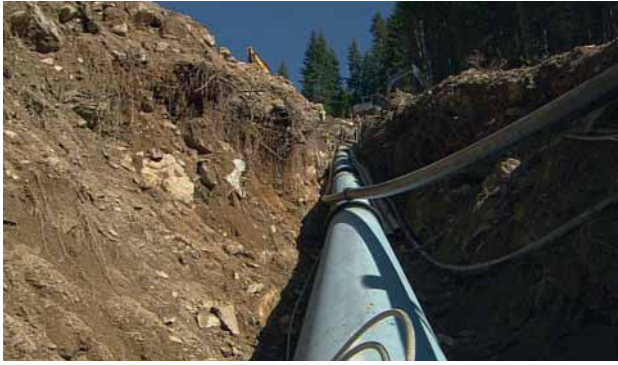
Fig. 5: Use of a cement mortar coated pipe in extremely difficult laying conditions
