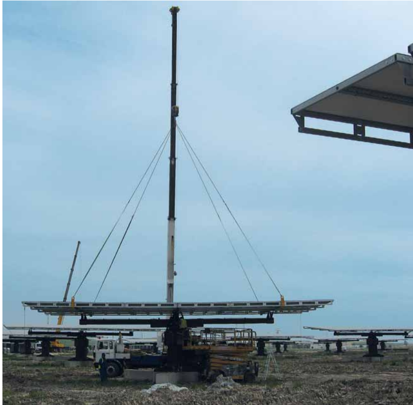
Fig. 10: A solar module being installed – this gives some idea of the size of an individual module, and hence of that of the solar energy park itself
