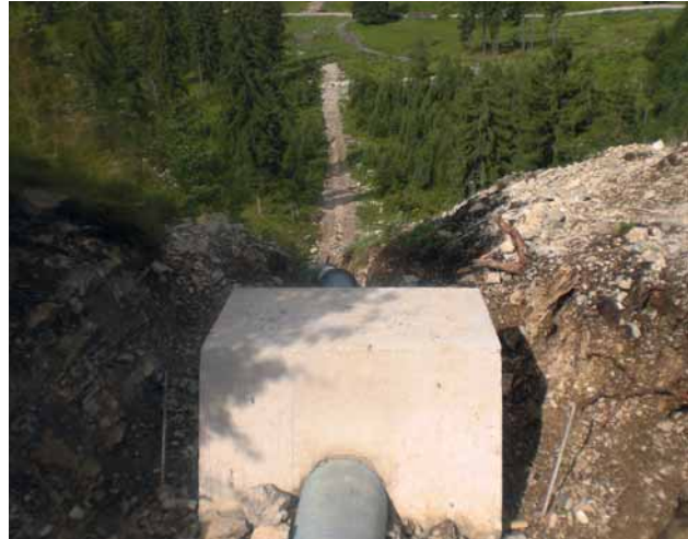
Fig. 15: A concrete thrust block to fix the top end of the pipeline in place on the steep slope
