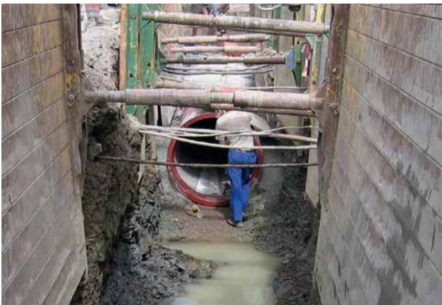
Fig. 5: The DN 1400 outer sewer from the rainwater overflow tank
