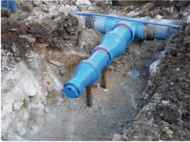
Fig. 11: Branch to a high level service reservoir
