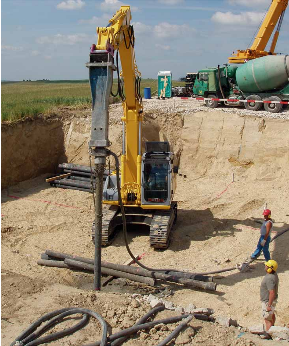
Fig. 4: Driving of a pressure-grouted ductile pile in practice, the example shown being a foundation for a wind power plant
