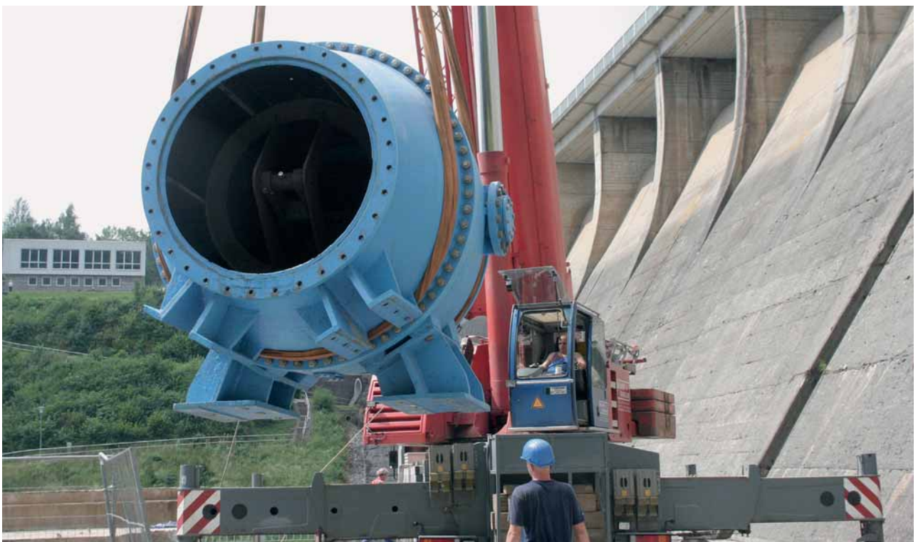
Fig. 3: The DN 2000 needle valve, weighing 40 t, has been removed from the dam and is being loaded.
