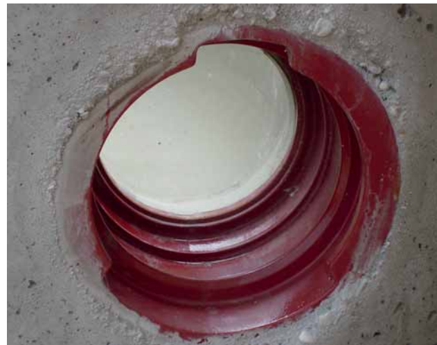
Fig. 5: Bottom section of concrete manhole with restrained VRS manhole connector
