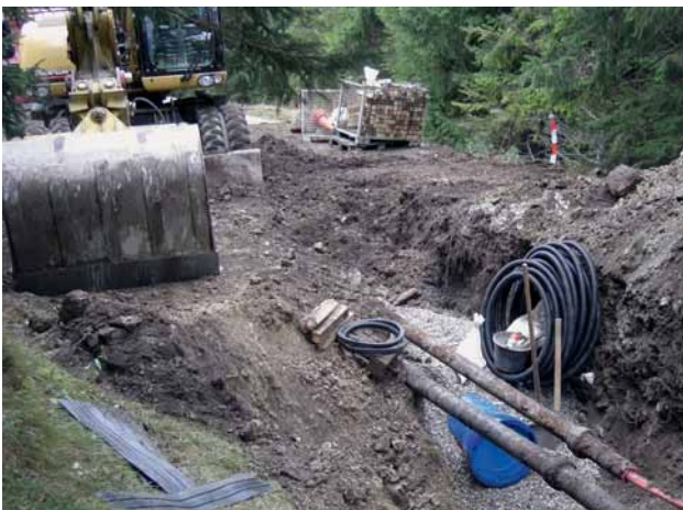
Fig. 3: The old water supply pipeline – two DN 100 drinking water pipelines of grey cast iron
