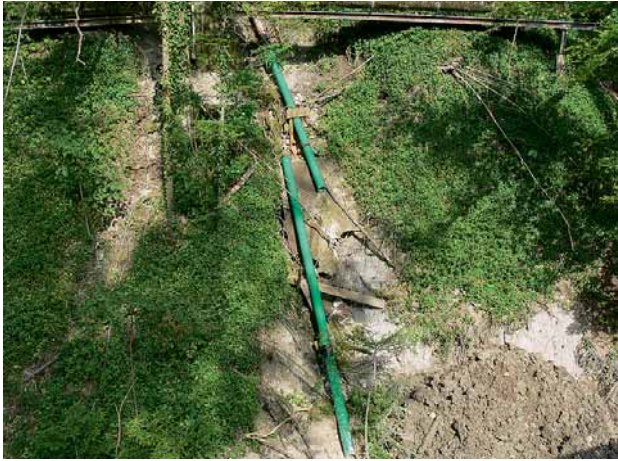
Fig. 2: Destabilised foundations which had slipped
