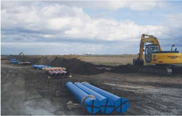
Fig. 3: DN 300 drinking water and sewer pipes laid out along the route where they will be installed in parallel
