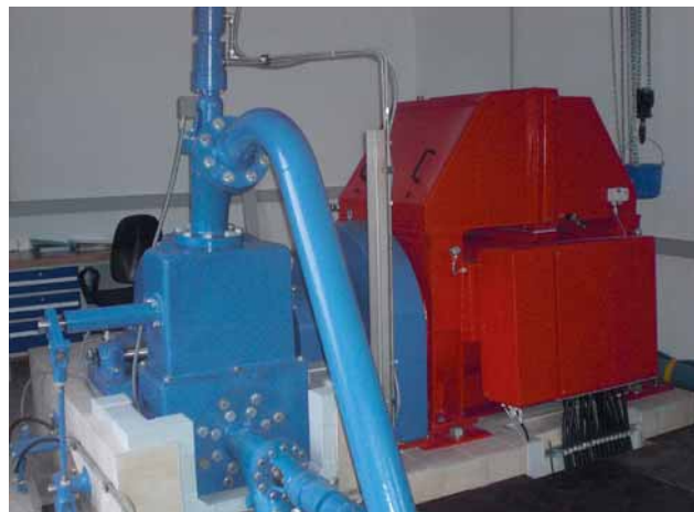
Fig. 5: The turbine and generator
