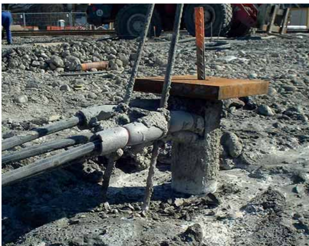
Fig. 5: A driven ductile pile pressure-grouted with concrete and its top pressure distributing plate
