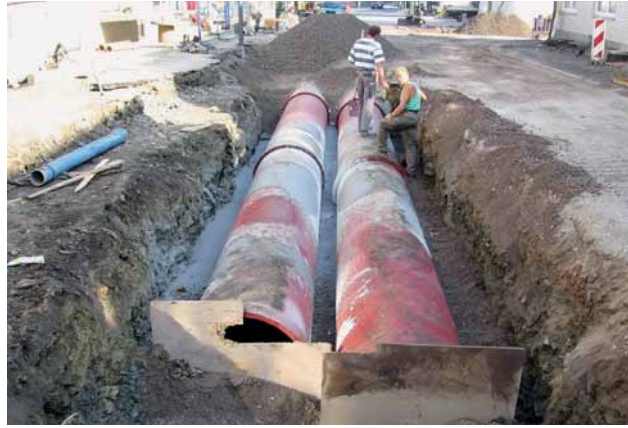
Fig. 6: Twin DN 1000 ductile iron pipelines forming the relief sewer from the overflow structure
