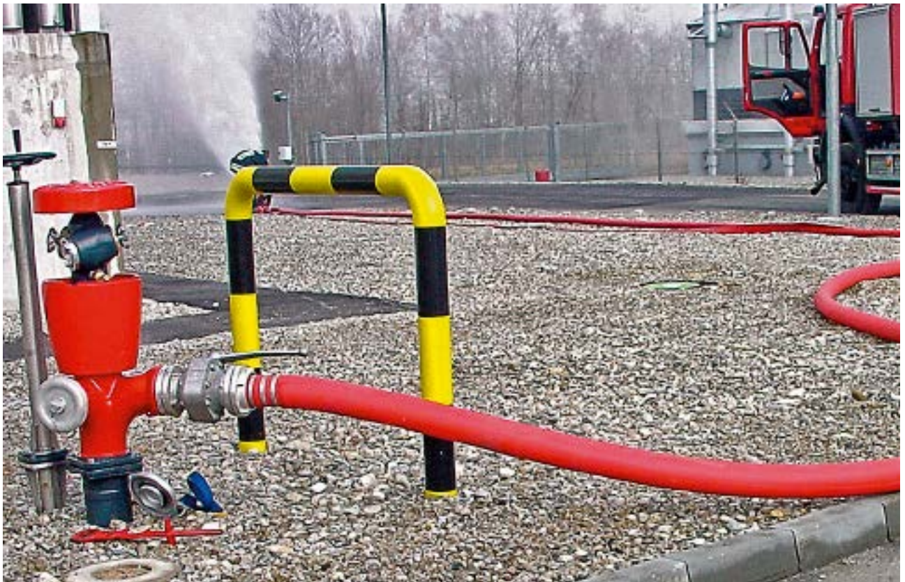
Industrial hydrant for extinguishing water supply on industrial premises
