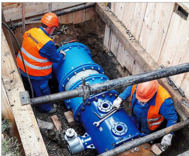
Figure 1: A view down onto the shutoff valve with block flanges on top
