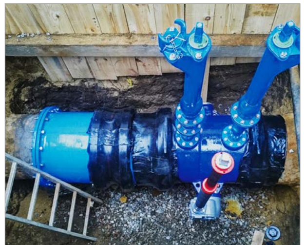
Figure 2: Installed shutoff valve with two underground hydrants
