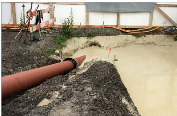
Figure 3: Immersing the wastewater pipes with cement mortar coating and BLS® push-in joints into the pre-drilled tunnel
