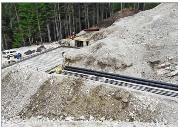
Figure 1: Filling and take-off pipelines to the future pumping station
