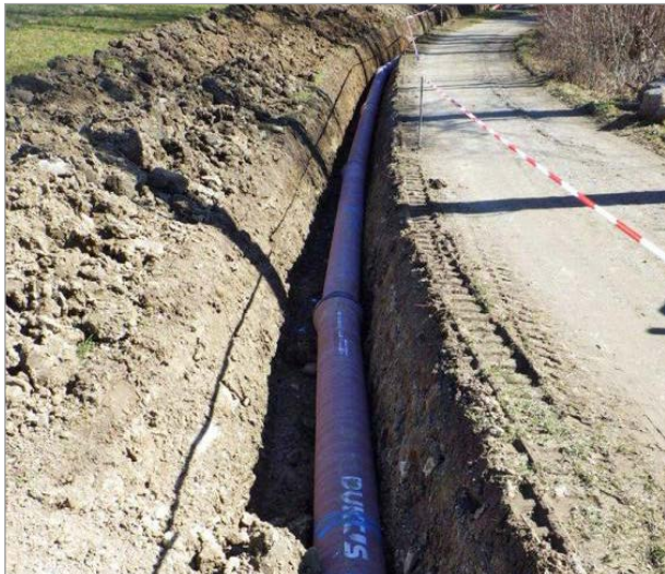
Figure 1: Installation of ductile iron pipes with cement mortar coating and BLS® push-in joints in the central section using the open trench technique
