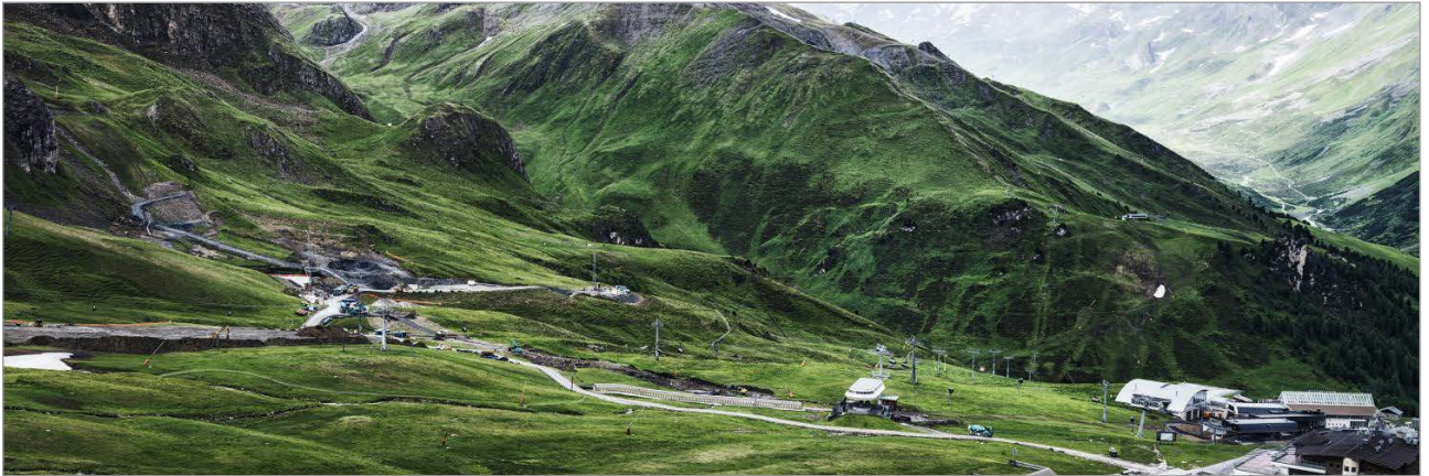
Figure 3: Panoramic view of the major construction site around the new Viderböden storage reservoir in the ski resort of Ischgl, Tyrol
