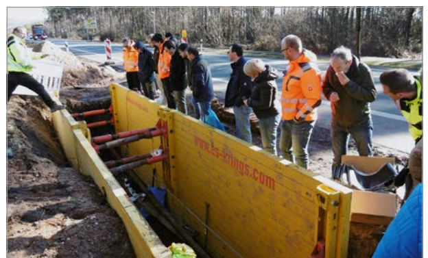
The installation of restrained ductile iron pipes and the burst lining technique is explained pit-side to an interested public.
