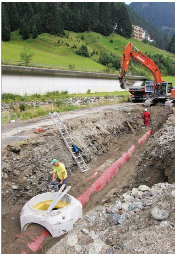
Backfilling the trench after installation of the manholes and the pipes with protection against extraneous water.
