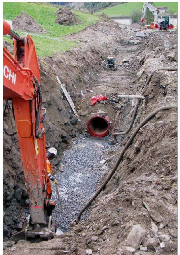
Installation of the ductile iron pipes in an area exposed to groundwater.
