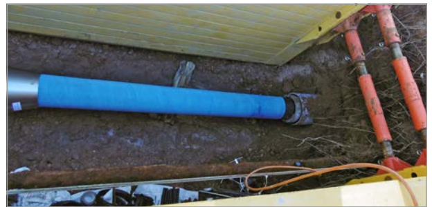
Bursting head with a DN 200 ductile iron pipe attached during the pulling-in process.
