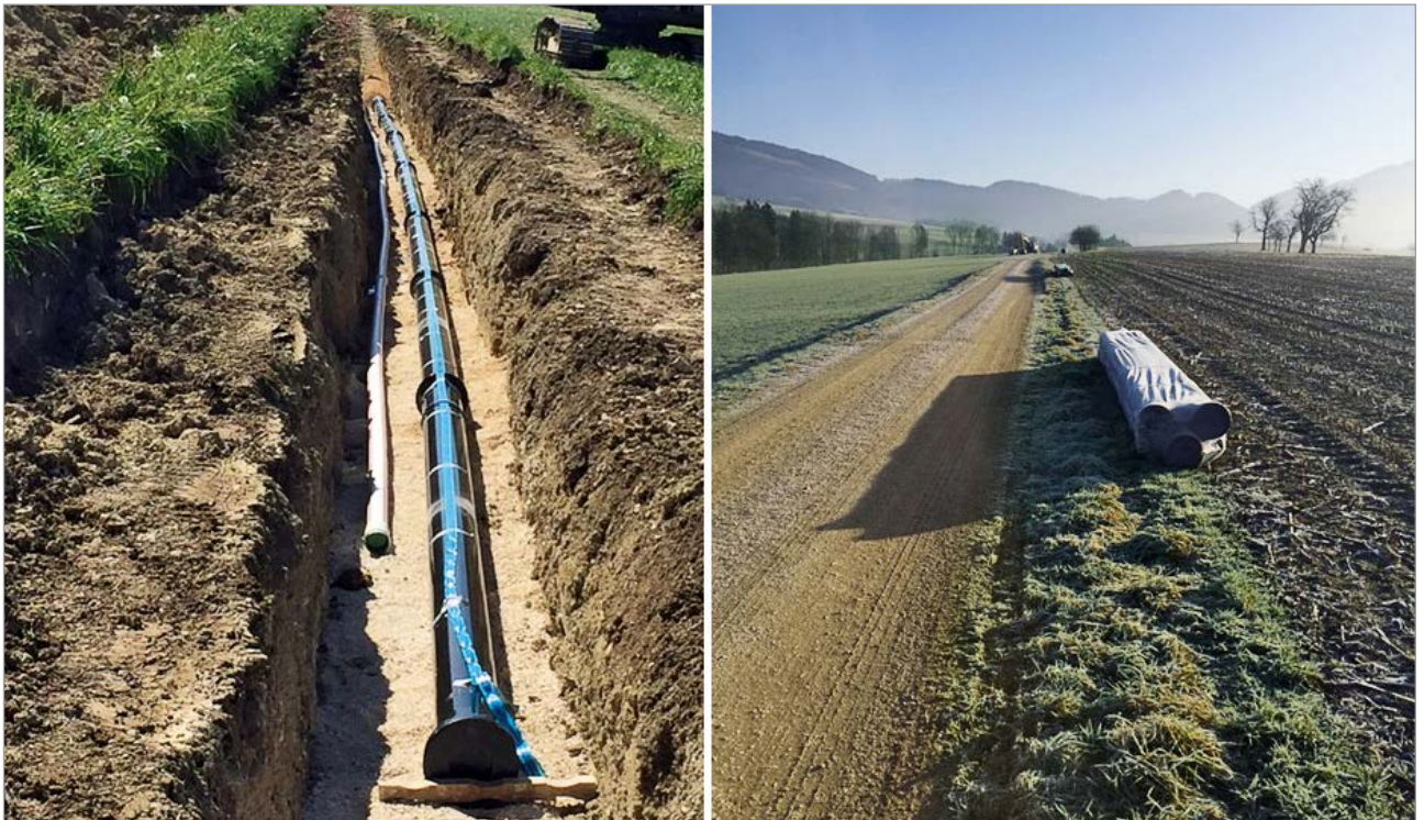
Transport pipeline between the villages of Mervelier and Vicques during installation work
