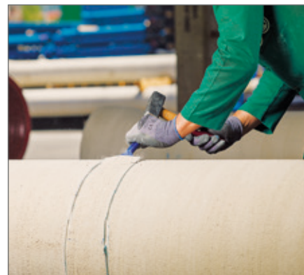
Once cut, the cement mortar layer can easily be taken out using a hammer and chisel.
