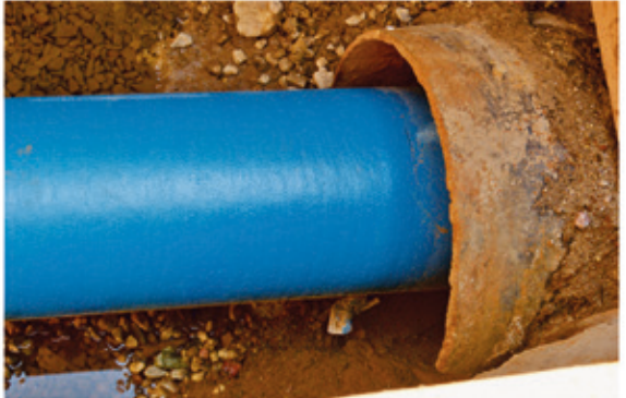
The pipe-string was pulled 6 m into the old pipeline in each case, dragging on the sheet steel cone.
