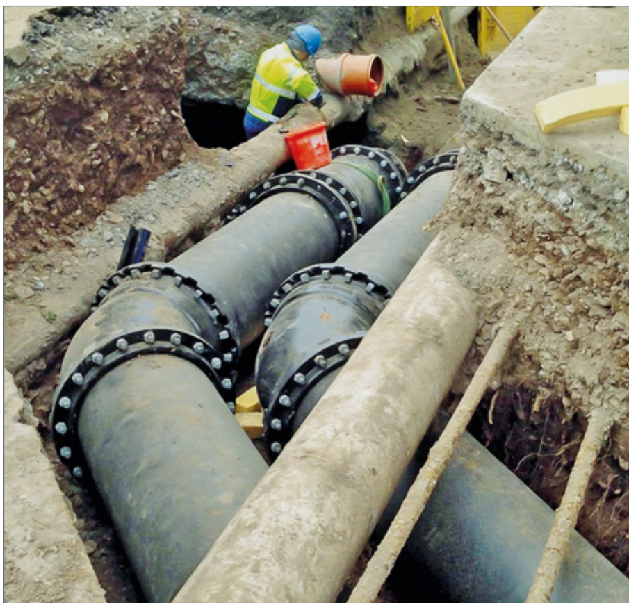
DUCPUR double DN 700 pipeline with feed and return flow.
