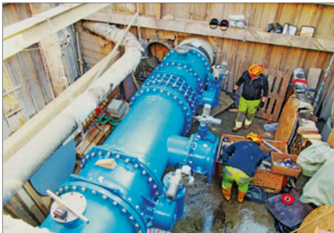
The use of Roco Wave butterfly valves from Erhard on a DN 1000 IWB pipeline in a modified valve pit.
