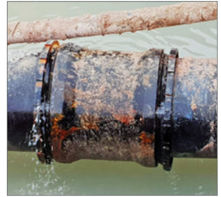
Leaking joint on a collar.
