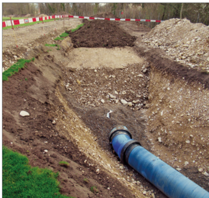
The different types of soil are clearly visible, but the ductile iron pipe with cement mortar coating is up to any situation. Unpolluted excavation material can also be used again for backfilling the trench.
