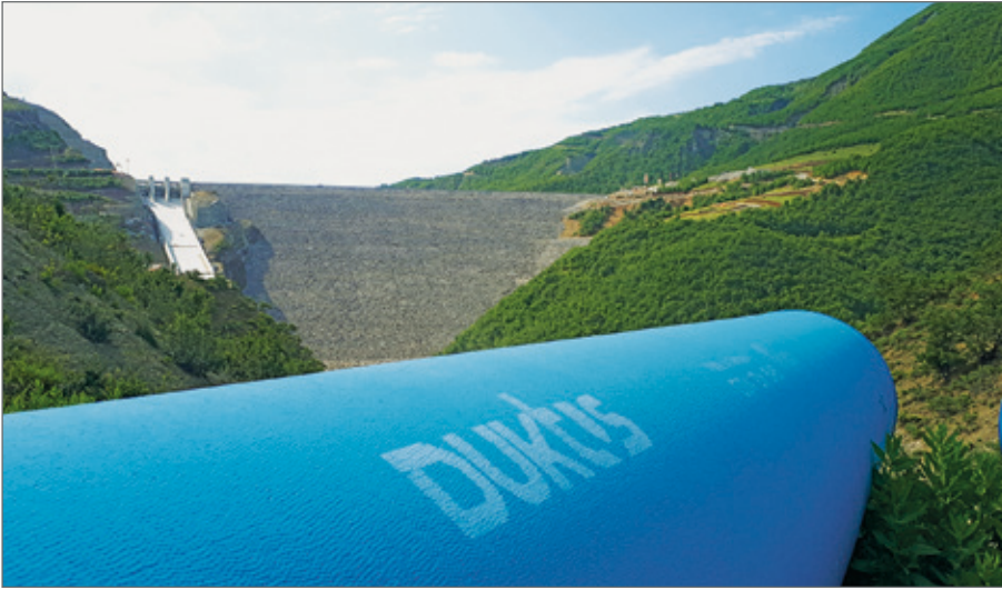
A view from the temporary storage area for pipes to the dam and emergency spillway.
