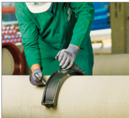
The cement mortar layer is partially removed for attaching the TRM tapping sleeve.
