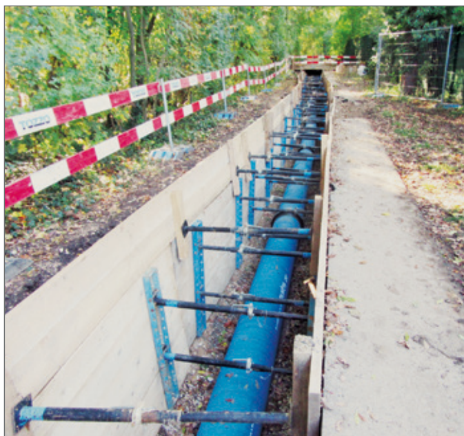
The pipes had to be installed under difficult conditions: tight access ways, narrow trenches and closely braced trench walls. Nevertheless, their installation went without problem.
