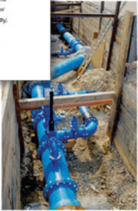
From time to time it was necessary to integrate valves and hydrants as well as branches and connections by open-trench installation.
