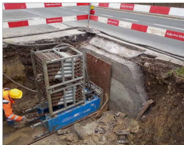
Figure 8: Bursting equipment in the main road with concrete thrust block and underpinning
