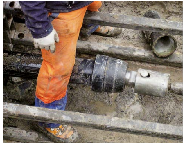
Figure 12: Traction head with ECOPUR pipe after 110 m of pipe pulling – emergence in the target pit
