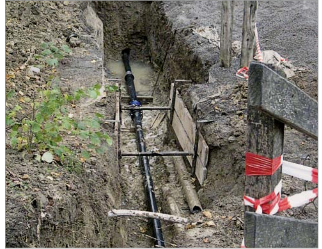
Figure 11: Connection of the pipes in the 1 st burst lining stage with the pipes installed using the open technique
