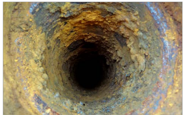
Figure 1: Grey cast iron pipe from 1930 with incrustations
