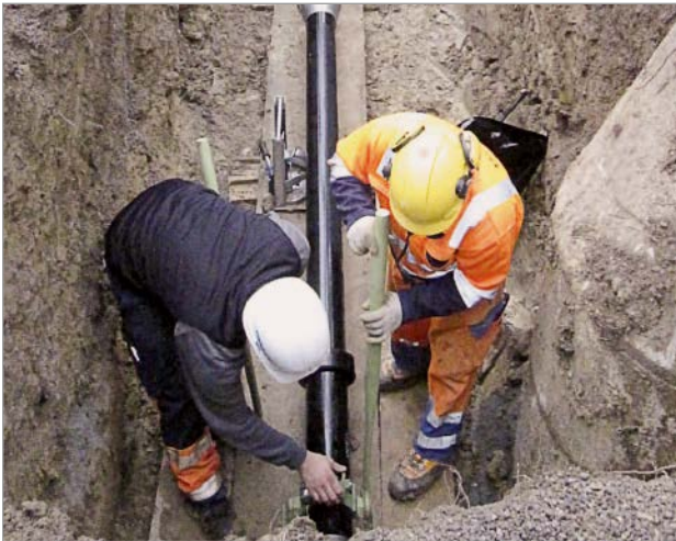
Figure 10: 1 st burst lining stage – underneath the play area and wild animal enclosure
