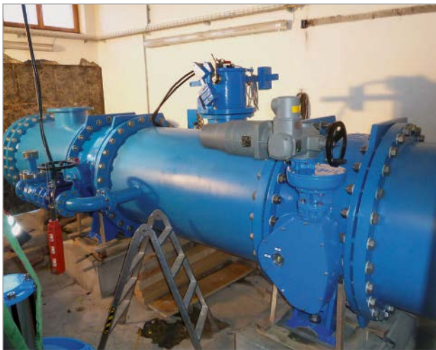
Figure 17: Apparatus room with pipe burst protection
