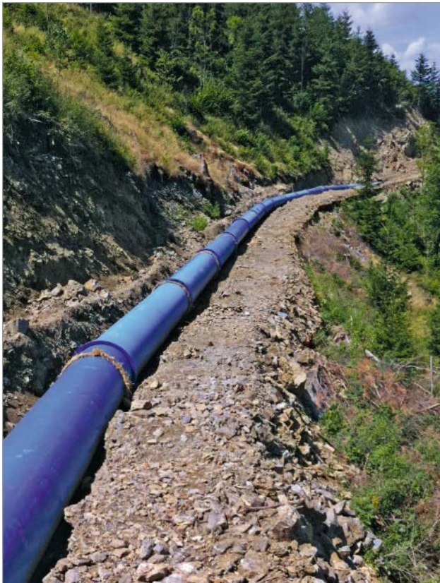
Figure 3: Newly laid DN 800 ductile iron pipes in the area of the Maria Kaltenbrunn spring
