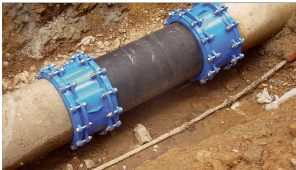
Figure 1: Closing up the old pipeline with a DN 500 ductile iron pipe section and two adapter couplings
