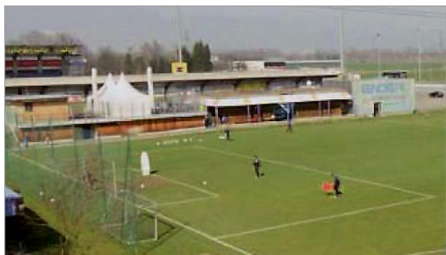
Figure 1: The SCR Altach football stadium – partial replacement of a water pipeline beneath the stands
