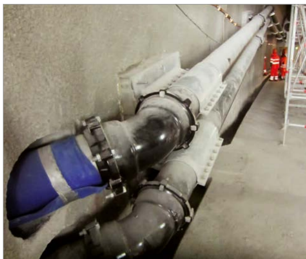
Figure 7: Wall penetration through the tunnel vault with fixed point consoles in the Tierfehd entry tunnel
