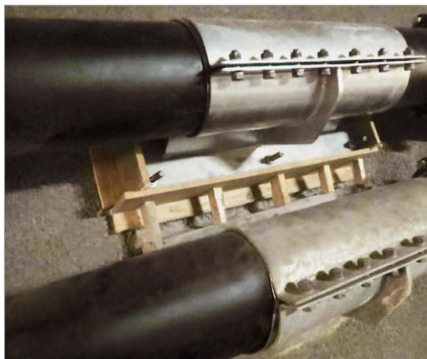
Figure 8: Formwork on the fixed point console for subsequent filling with liquid mortar
