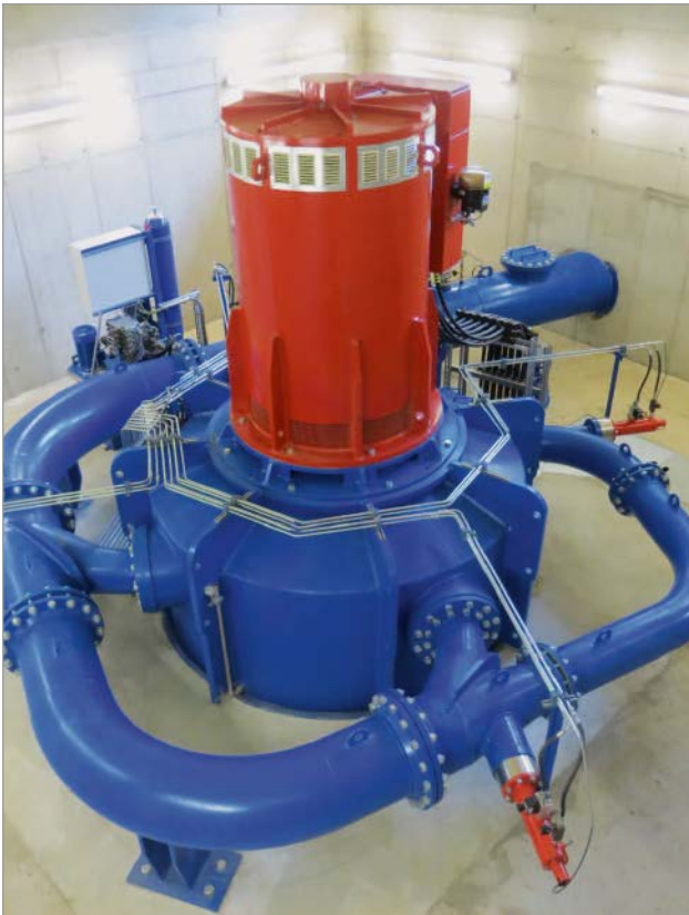
Figure 2: Four-jet GHE Pelton turbine equipped with a Hitzinger synchronous 3-phase generator
