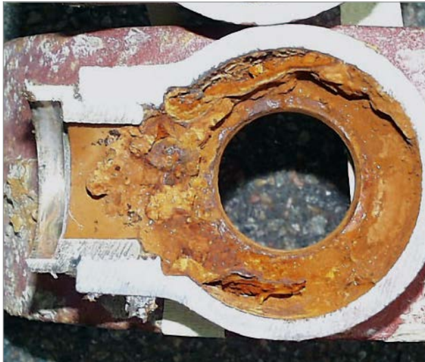
Figure 2: Corrosion in the threaded area of a domestic connection valve
