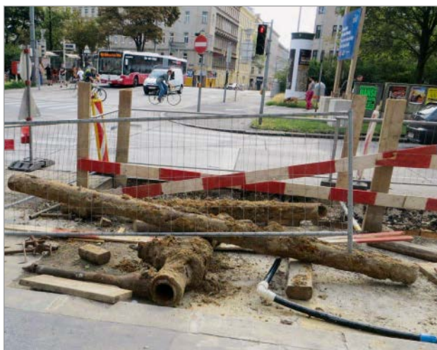
Figure 1: Replacement of iron pipes more than 100 years old in the area of the Hernalser ring road
