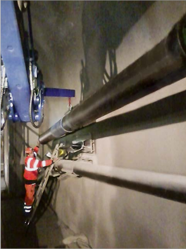
Figure 12: Assembly of ductile iron pipes with a mini-digger in the sloping tunnel
