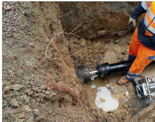
Figure 7: Starting the pipe-pulling – upsizing head and traction head with traction force measurement
