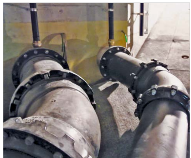
Figure 6: Connection of collecting tank at tunnel metre TM 1,213
