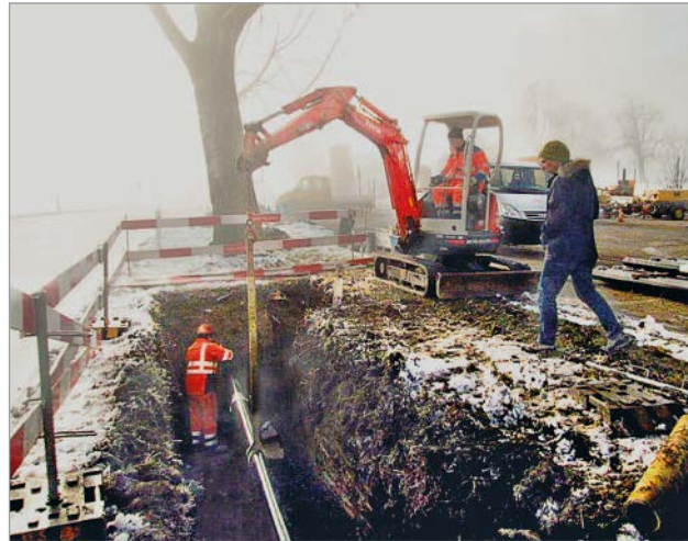
Figure 6: Lowering the pipe into the launch pit in Albisstraße – burst lining in the area of the avenue of trees
