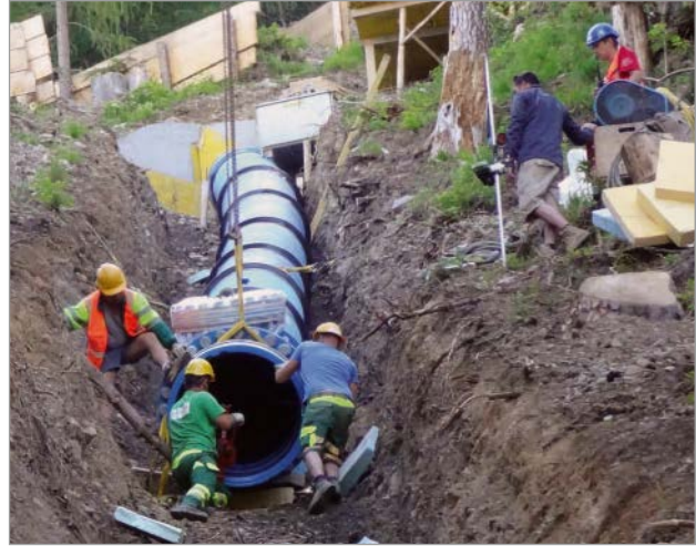
Figure 14: Pipe assembly going downwards
