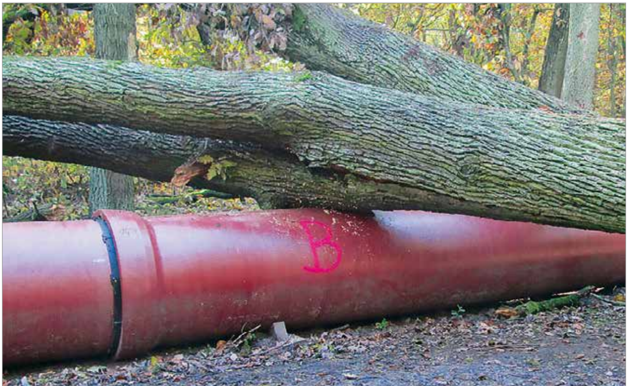
An uprooted oak tree which fell onto the interim pipeline did not result in any operational disruptions
