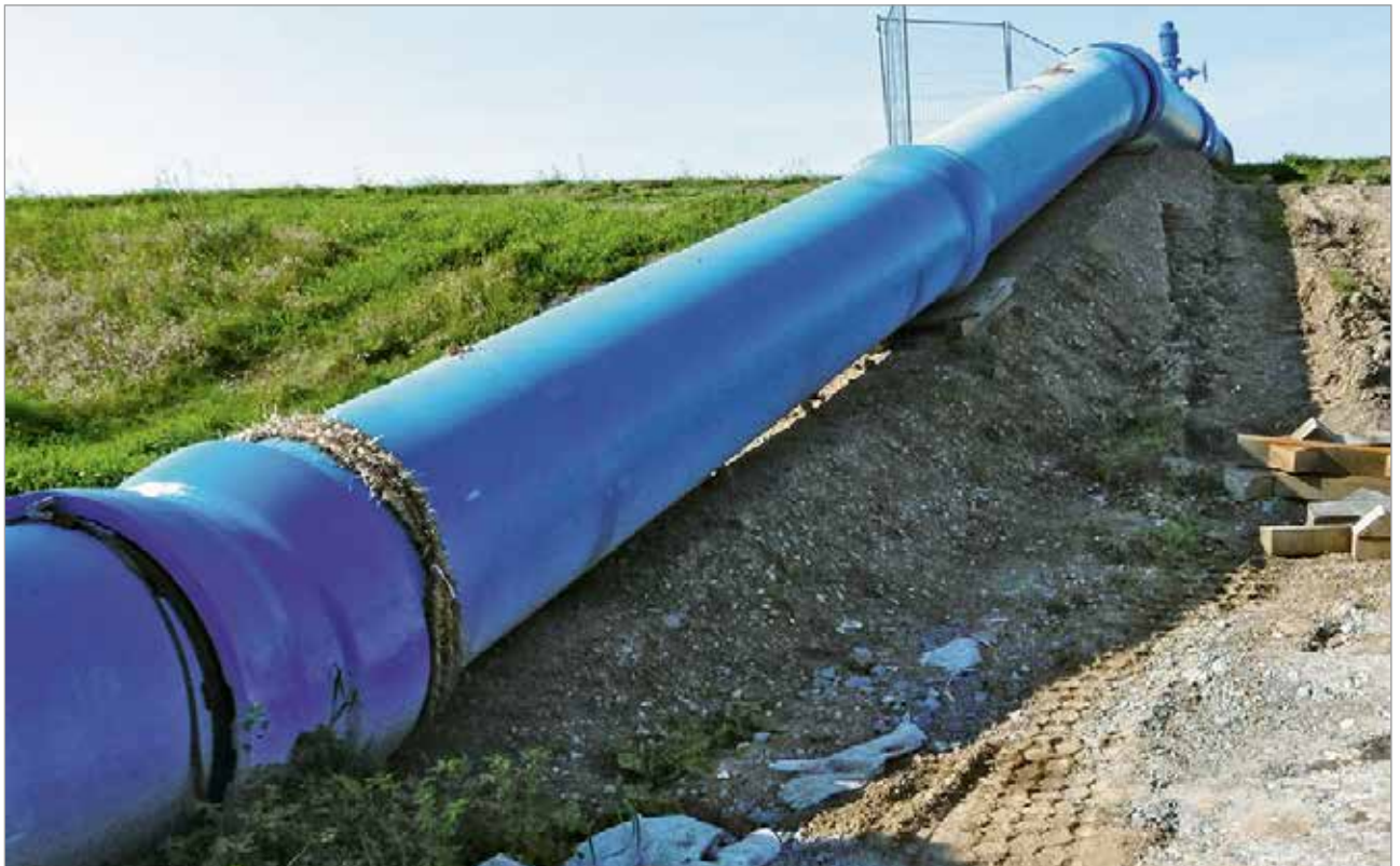
The route of the DN 800 interim pipeline over the dike between the pipe bridge over the River Mulde and the Canitz waterworks
