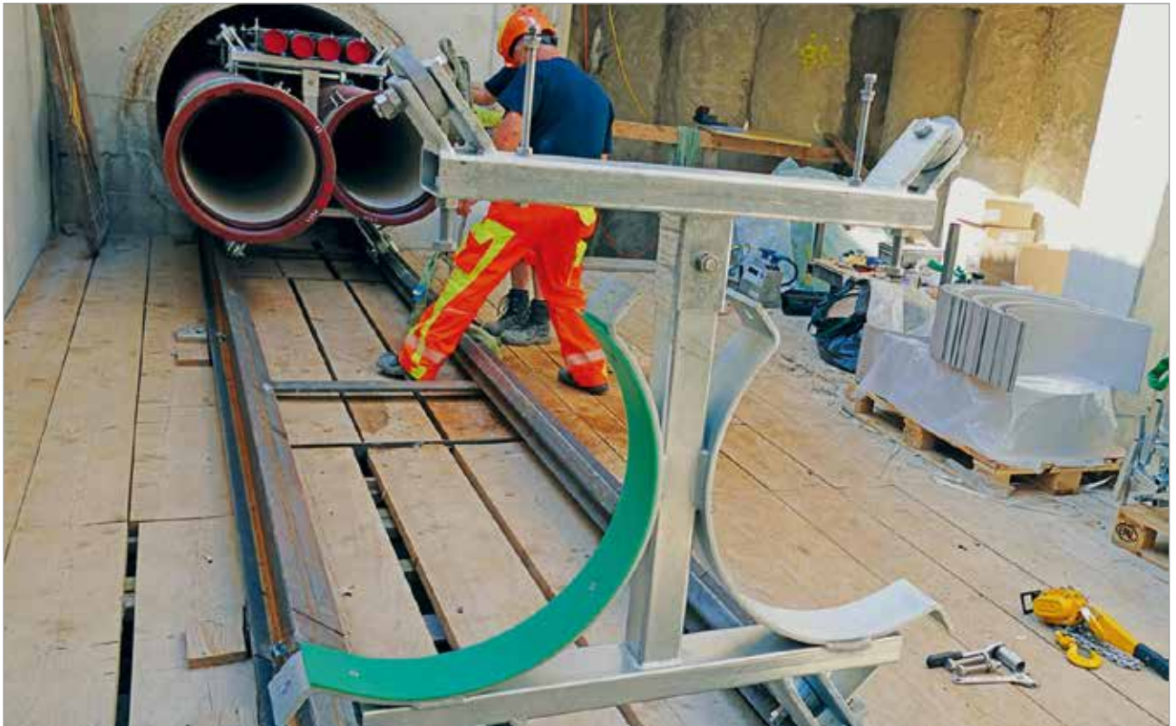
Pulling-in of two cast iron pipes simultaneously using specially developed mobile double pipe clamps.
