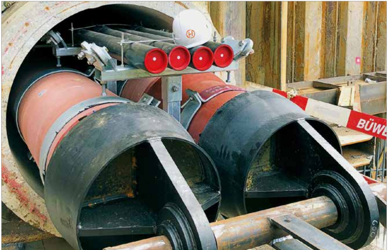
Arrival at the target shaft. The extremely tight space conditions in the microtunnel are clear to see.
