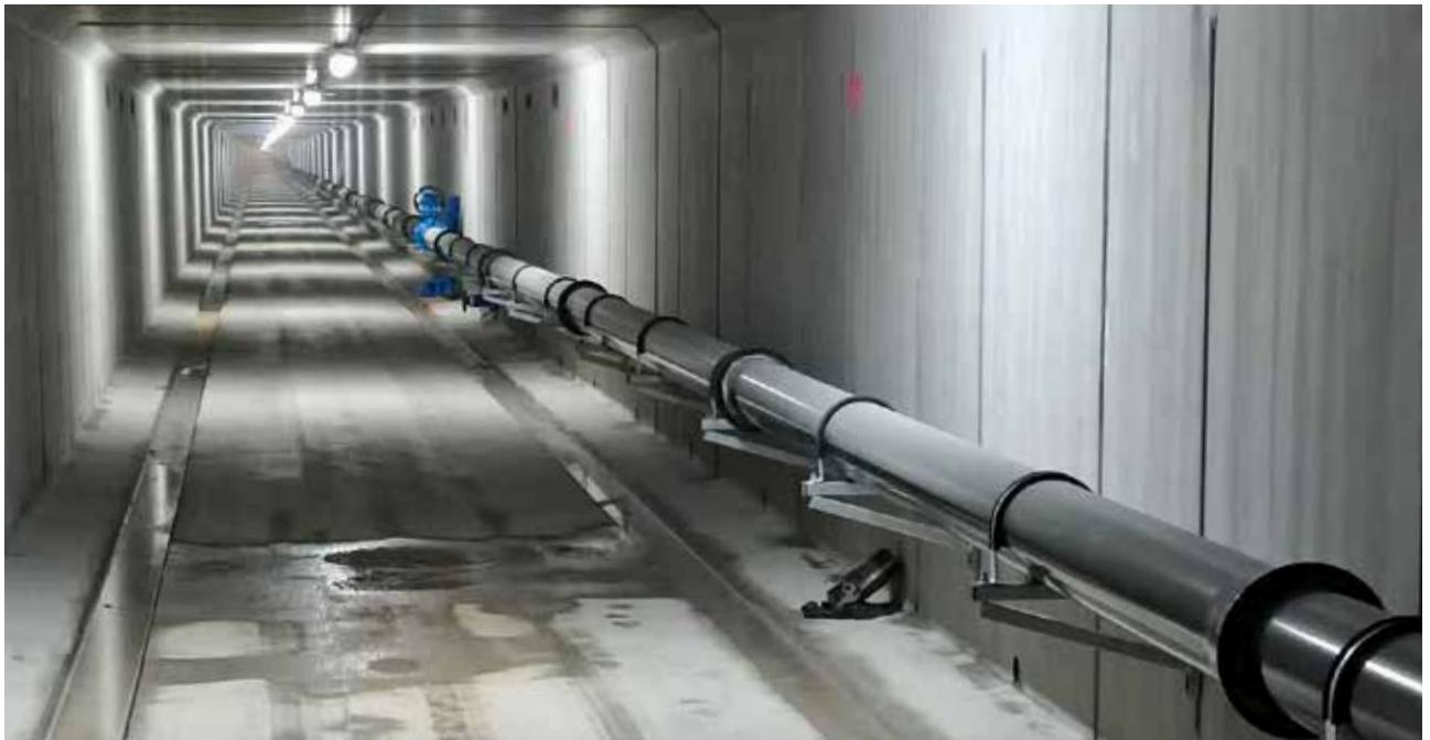
The service duct beneath the 3 rd tube of the Belchen tunnel.
