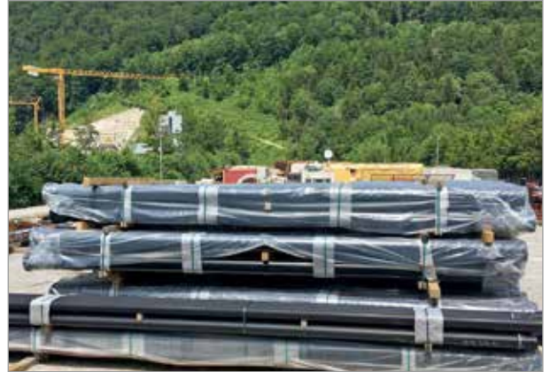
vonRoll ECOPUR ductile iron pipes before their installation in the service duct.
