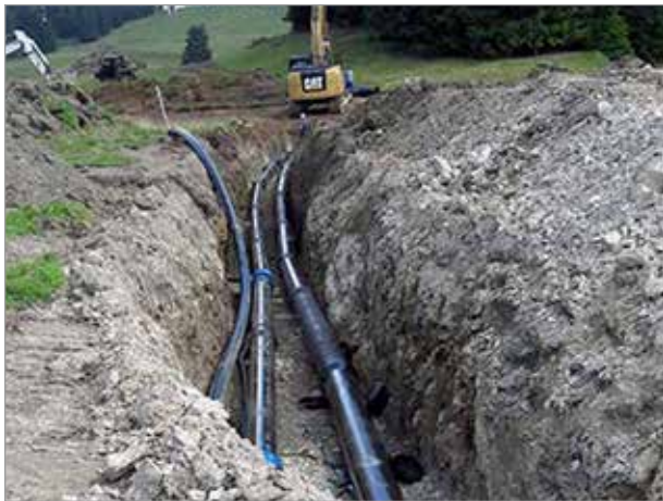
Careful installation of ductile iron pipes in a new trench for the Zinsberg cable railway
