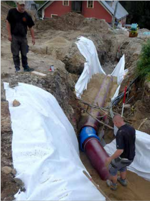
A 30° change of direction of the power station pipeline in Seebachschleife with a MMK 500/30° fitting and BLS® socket joints, lined and coated with epoxy blue.
