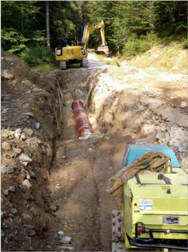
Once the ductile iron pipes had been laid alongside a forest road, the backfill material is compacted layer by layer.
