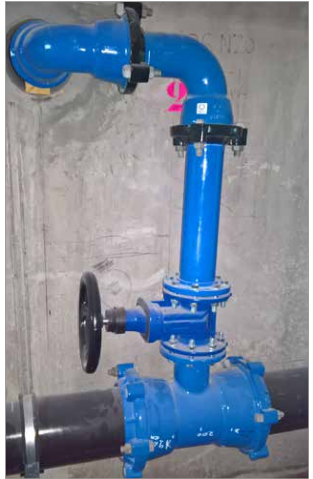
vonRoll VS 5000 shutoff valve in the service duct.
