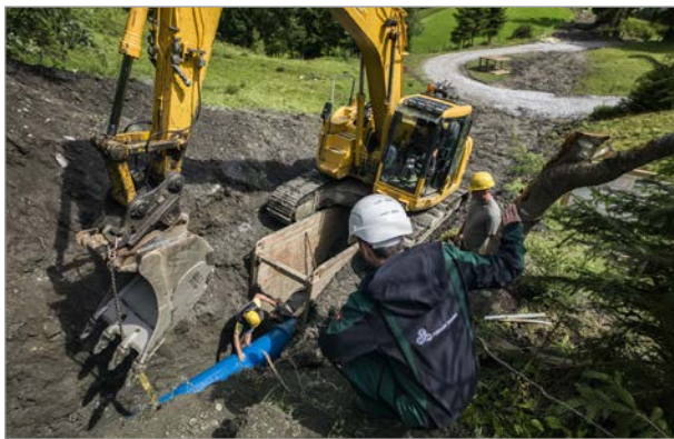
Assembling the pressure pipeline with VRS®-T restrained push-in joints in the pipe trench
