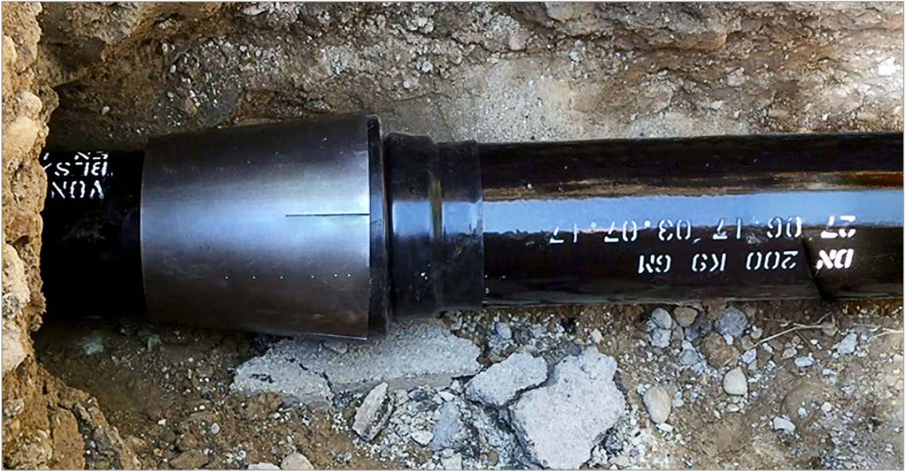
Pulling the ECOPUR ductile iron pipes into old grey cast iron pipeline after bursting
