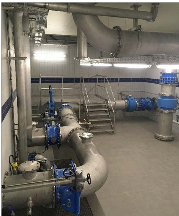
Pipe basement in the Hattgenstein water tower with ERHARD ROCO wave butterfly valves in the background with a hydraulic drive and built-in adaptors and spacers.
