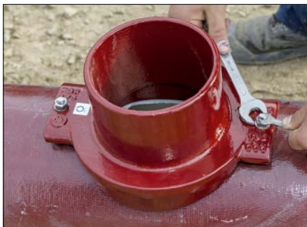
Fig. 19.33: The connection branch is positioned and then fixed to the ductile iron pipe with retaining screws
