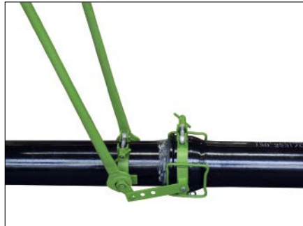
Fig. 19.21: Example of assembly equipment for pulling ductile iron pipes \leq \text{DN } 300 together
